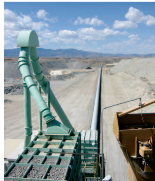
Figure 58. Primary crusher (foreground) and blending hall (at distance) at Holcim's Portland cement plant in Florence. The long belt connecting the two is necessitated to ensure proper blending of limestone, shale, and sandstone into a clinker mix in the blending hall.
