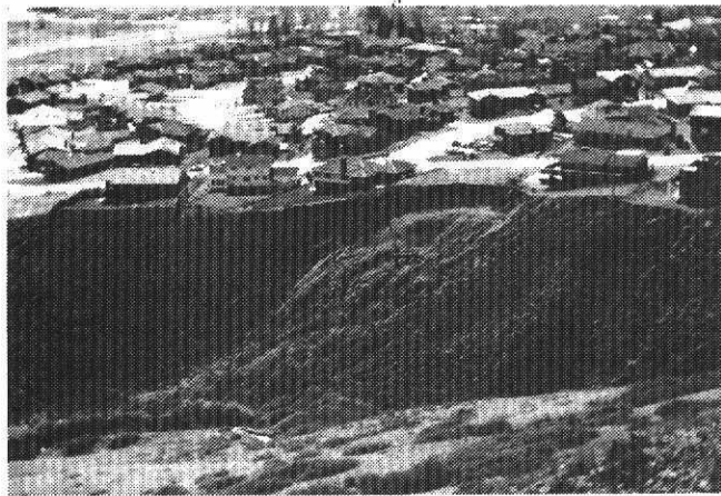
Figure 10b. Rotational landslide, Golden, Colorado (photograph by Colorado Geological Survey).
