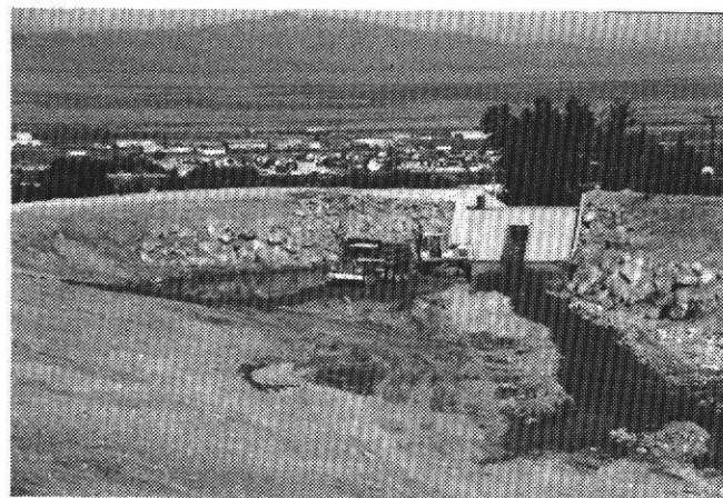
Figure 26. Rudd Creek debris basin in Farmington, Utah constructed in 1983–84 (photograph by Robert Kistner, Kistner and Associates).
