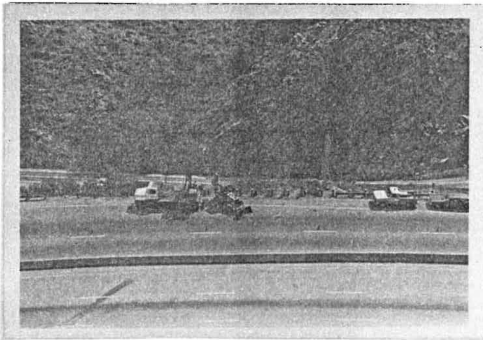
12. View showing equipment in use at site. The back hoe is used to lift the wood posts and position them under the post driver hammer.
