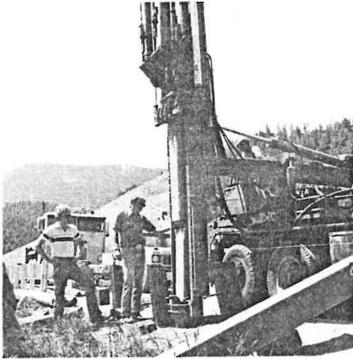
11. The post driver is shown driving a wood post. Due to damage to top of post, subsequent posts were driven using a steel cap on the top of the post.
