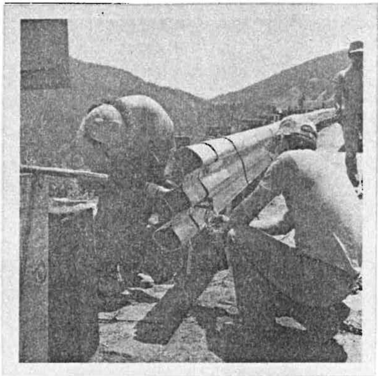
14. Straight internal splice sections were used to connect the tubular thrie beam sections.
