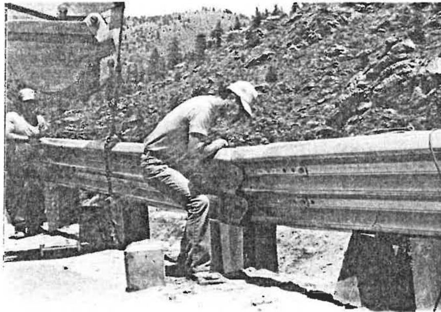
13. Back hoe being used to support tubular thrie beam as the beam sections are being joined.
