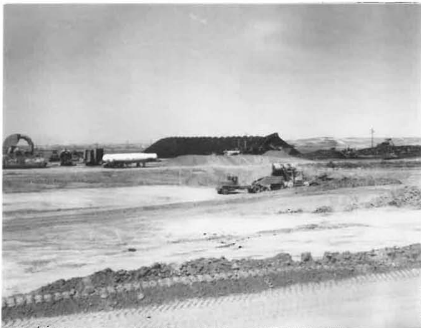
Photograph No. 4 Pavement stockpiled at plant site. Dozer is working old pavement (right), crushed pavement stockpile (center), and start of virgin aggregate stockpile to right of propane tanks.
