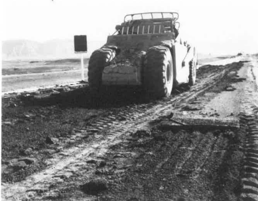
Photograph No. 2 Scrapers picked up alternate six foot wide strips. Only scraper teeth entered base course.
