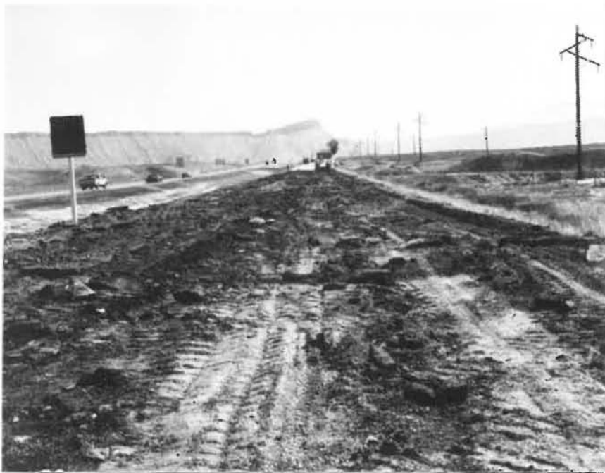
Photograph No. 3 Base following pavement removal by scrapers. The remaining pavement was windrowed and picked up using a front end loader.
