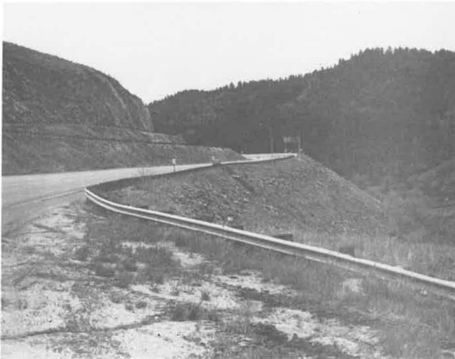
Long distance view of the Mt. Vernon Canyon Runaway Truck Escape Ramp. The overhead sign marks the beginning of the approach.
