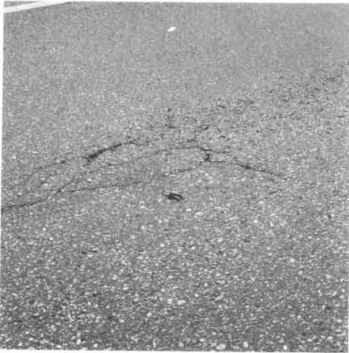
Closeup of Alligator cracks beginning to appear in Section 3.
