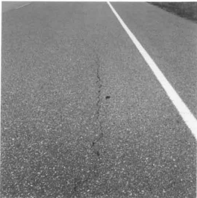
Typical longitudinal cracks observed in Section 3.
