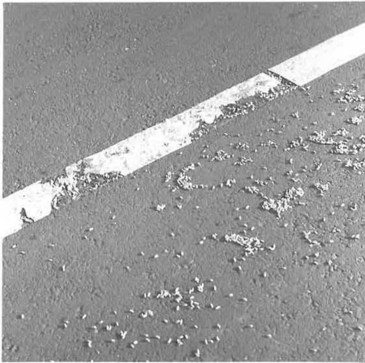
Marking bladed off of rough spot in pavement. Some pavement pulled off with marking material.
