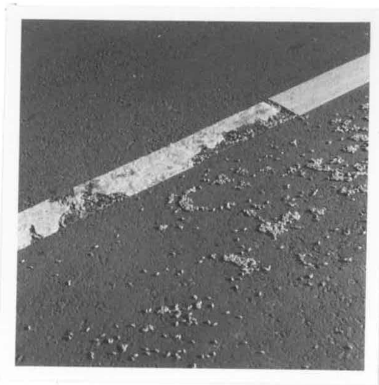
Striping bladed off at rough spot on pavement. Some asphalt pavement was pulled off with the striping material.
