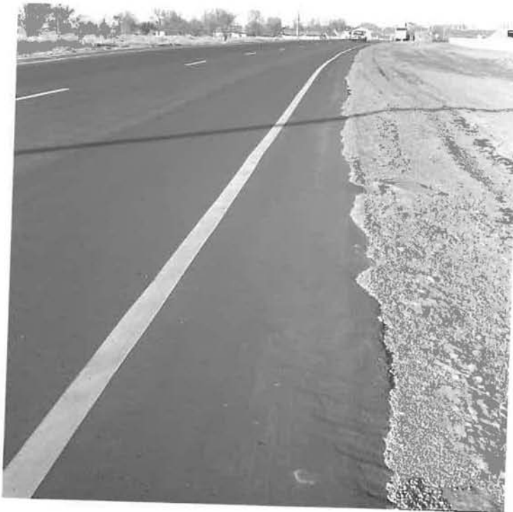
Inside lane yellow stripe on asphalt pavement. In good shape and not showing any evidence of wear or deterioration.
