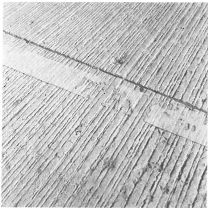
High spots in the concrete pave- ment allow the snowplow blade to wear off the striping material.
