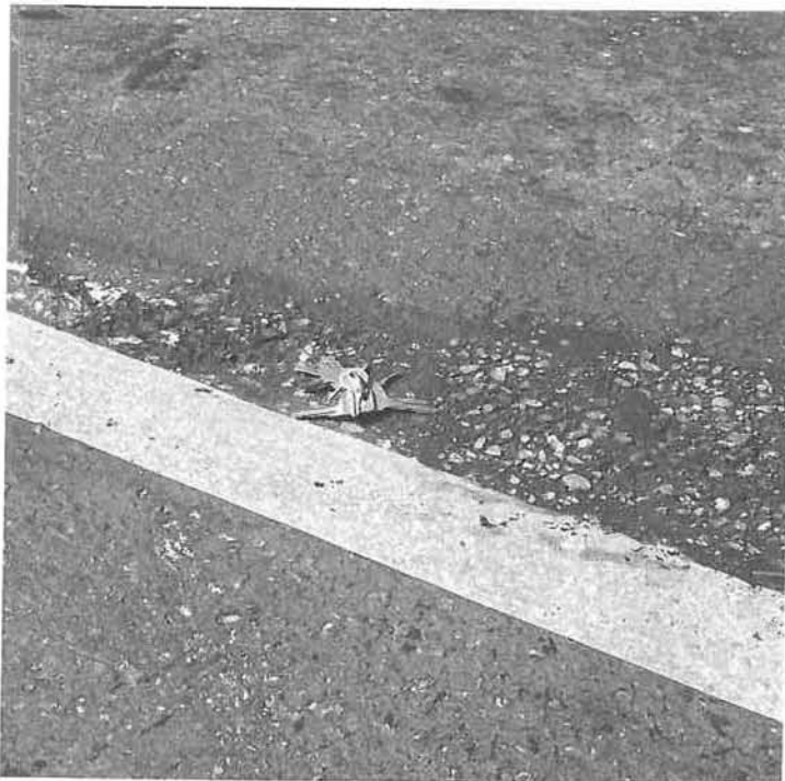
Yellow edge line which was applied over a rough section of pavement. Damage occurred shortly after application.
