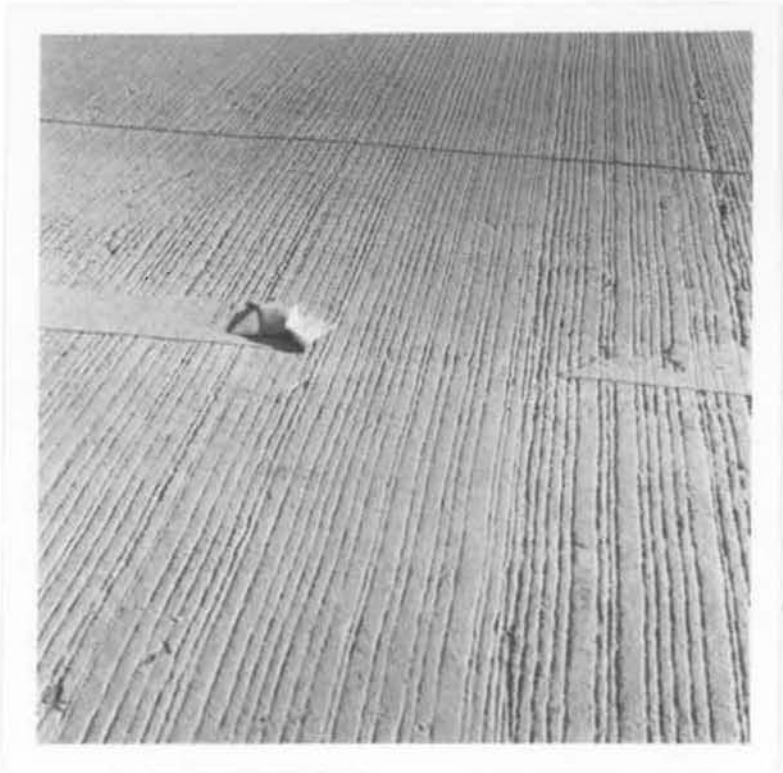
Centerline striping where the snowplow blade picked the edge of the striping and peeled it off.
