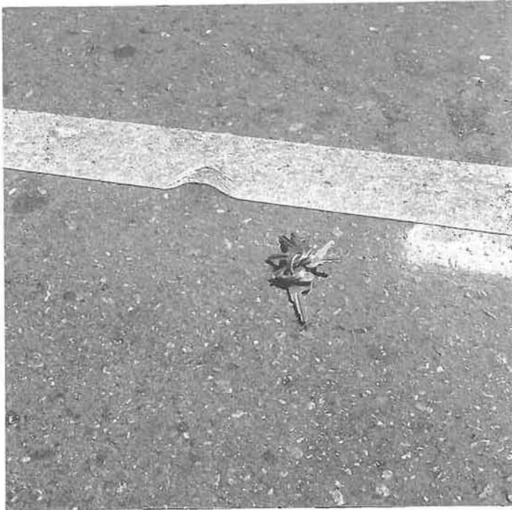
Yellow edge line which had received damage and discoloration shortly after being applied.
