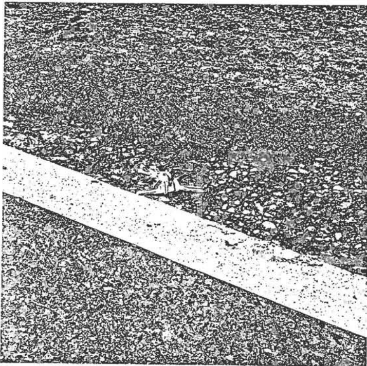
Yellow edge line which was applied over a rough section of pavement. Damage occurred shortly after application.
