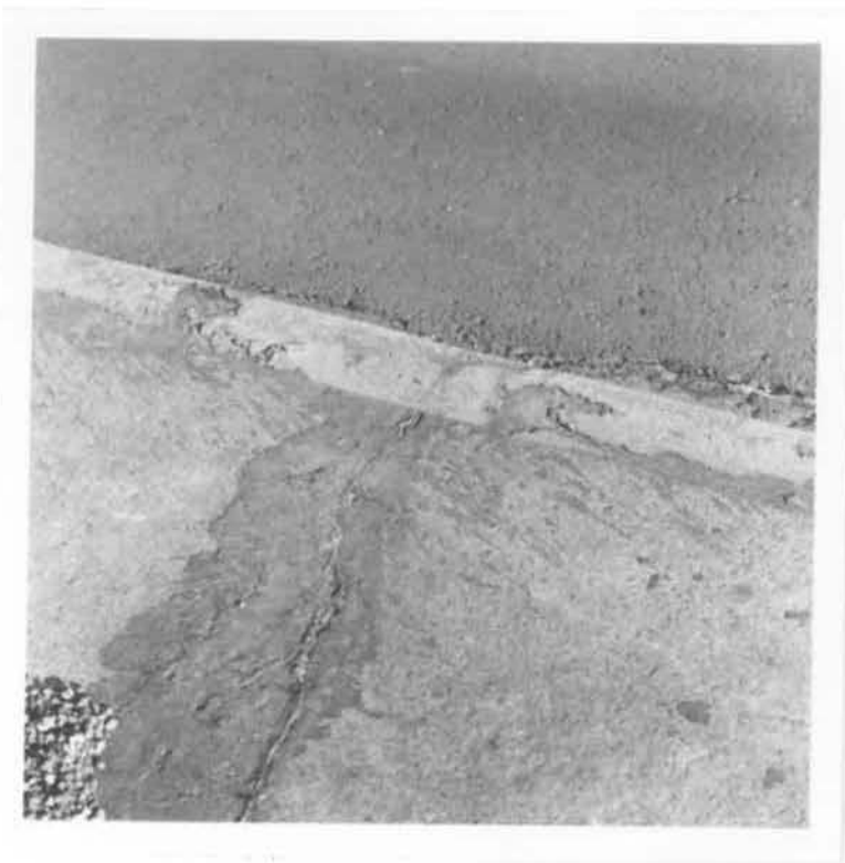
Striping worn off by snowplow blade at high spot on pavement.
