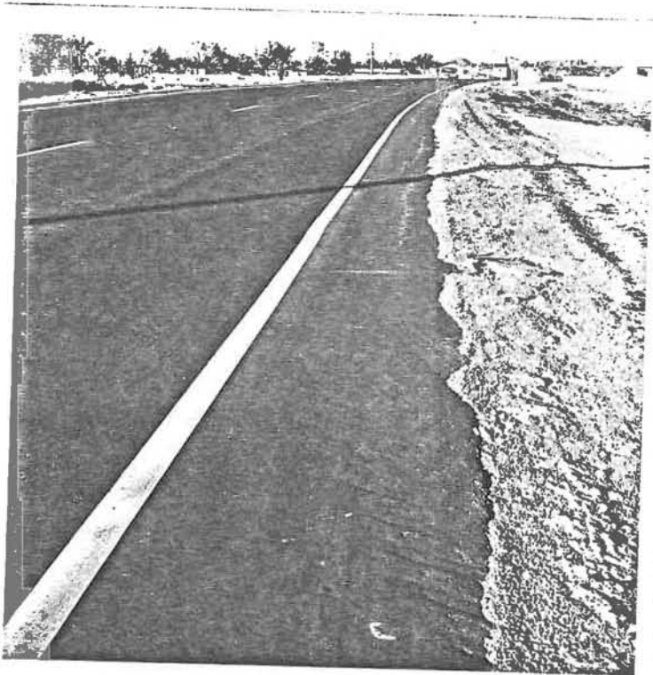
Inside lane yellow stripe on asphalt pavement. In good shape and not showing any evidence of wear or deterioration.
