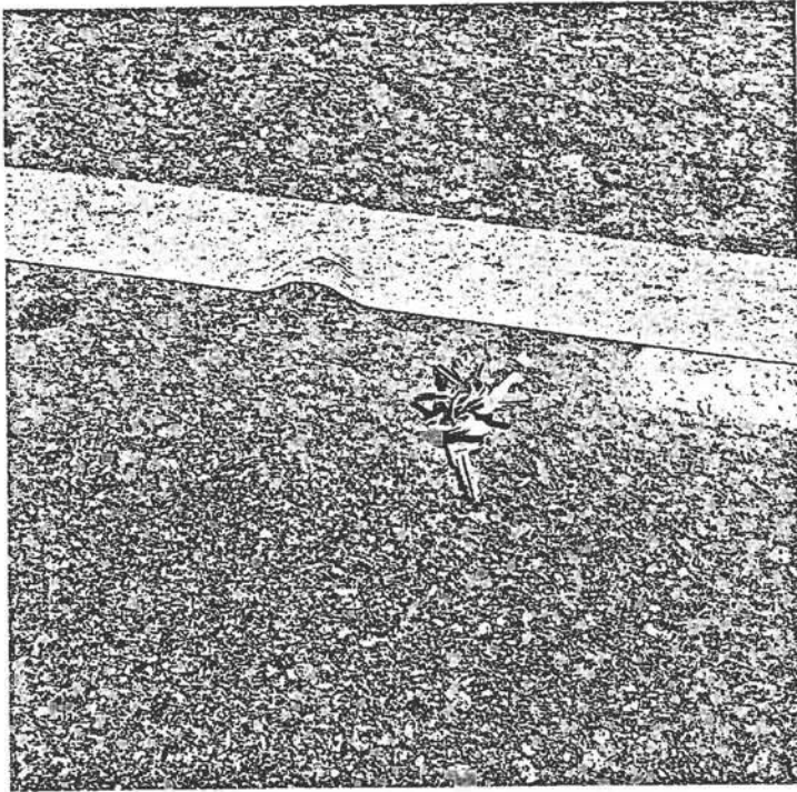
Yellow edge line which had recieved damage and discoloration shortly after being applied.
