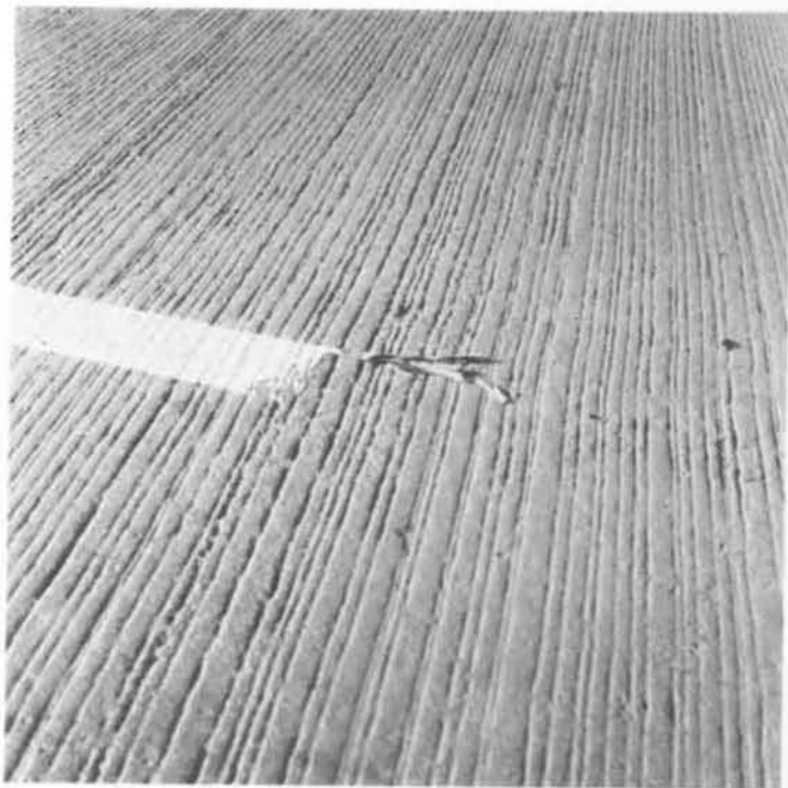
Area where the snowplow blade has peeled back the striping.
