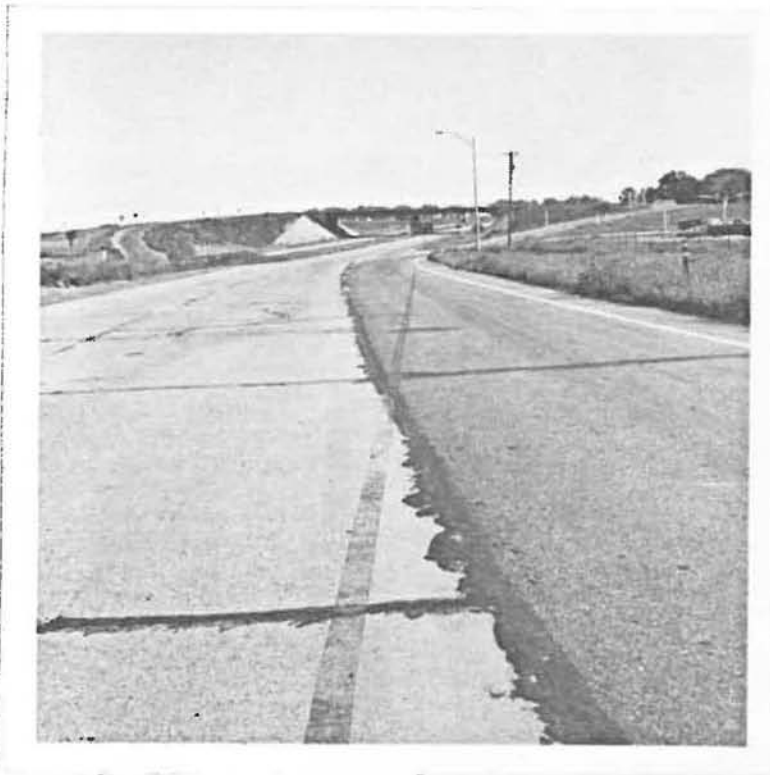
Area where some residue remains after removal of marking material.
