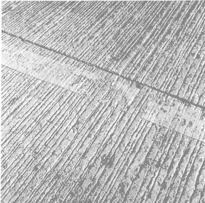
High spots in the concrete pavement allow the snow plow blade to wear off the pavement markings.
