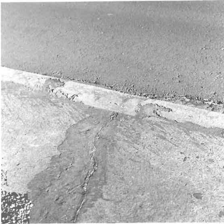
Marking worn off at a high spot.
