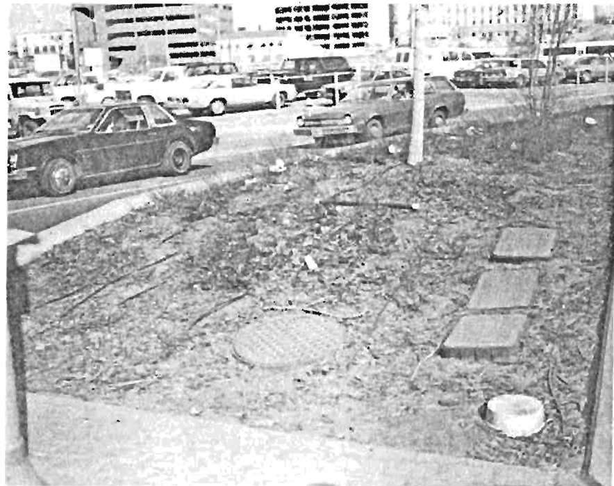
Tubing and manifold piping exposed. This area is adjacent to pedestrian walkway. The mulch has been stripped away.
