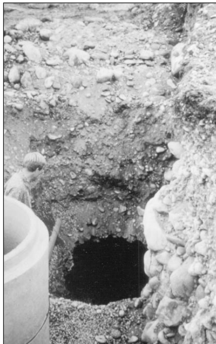
Subsurface void encountered during construction in river terrace gravel overlying Eagle Valley Evaporite—
