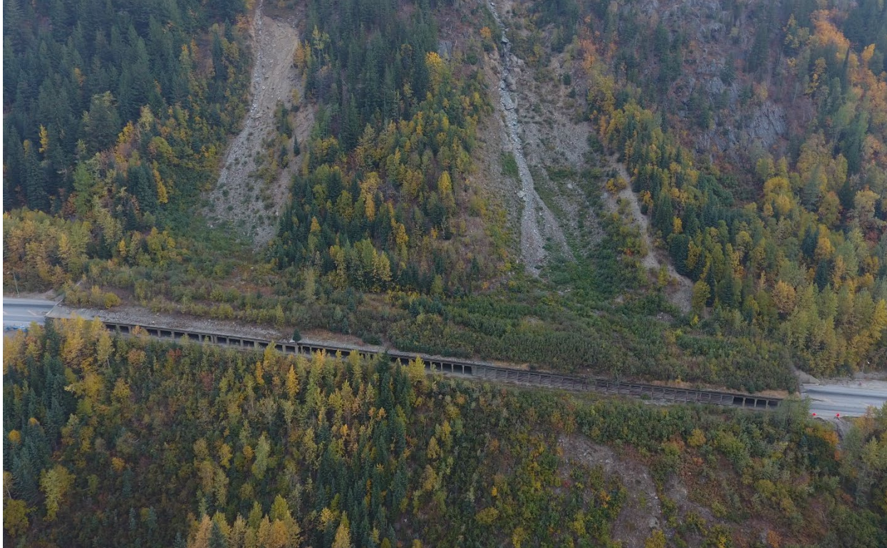
Figure 37: Debris and vegetation accumulation on top of the combined Tupper #1 (right) and Pioneer (left) snow sheds observed in 2017. A major shed rehabilitation program by Parks Canada has removed this debris and improved the management of surface and subsurface water (Photo: Dynamic Avalanche Consulting).
