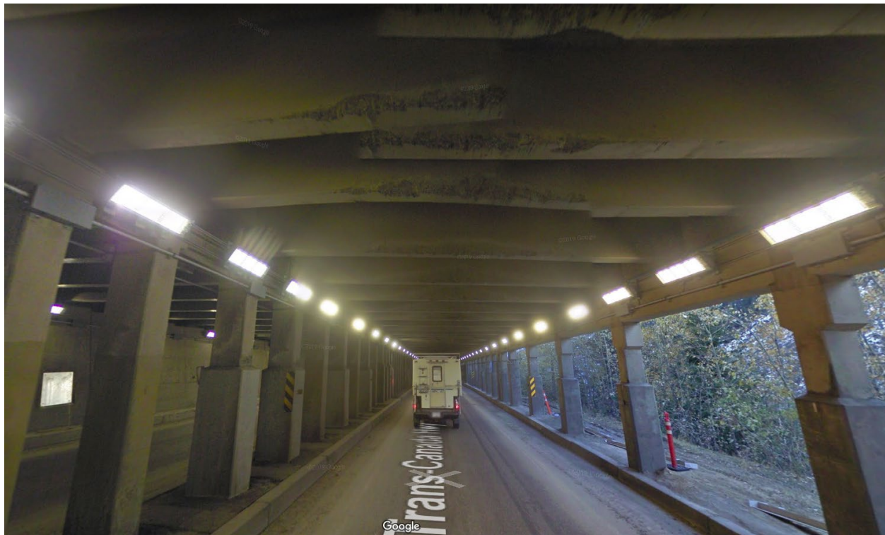
Figure 32: Overhead damage to the Tupper #1 snow shed has occurred where the original metal arch-shaped Pioneer shed joins the flat-roofed concrete Tupper #1 shed (Photo: Google Earth, 2020).
