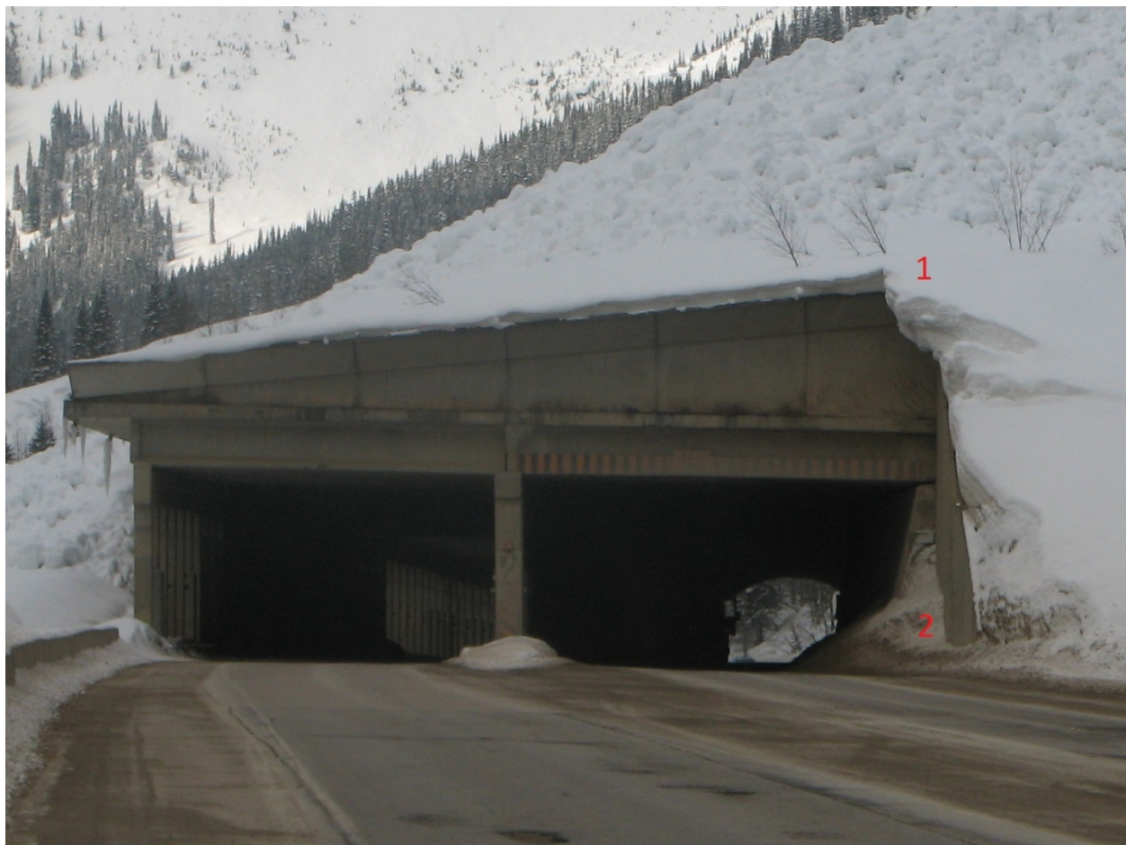
Figure 35: Two snow shed maintenance issues: (1) overhanging cornice snow and (2) snow accumulation at the portal (Photo: Alan Jones)
