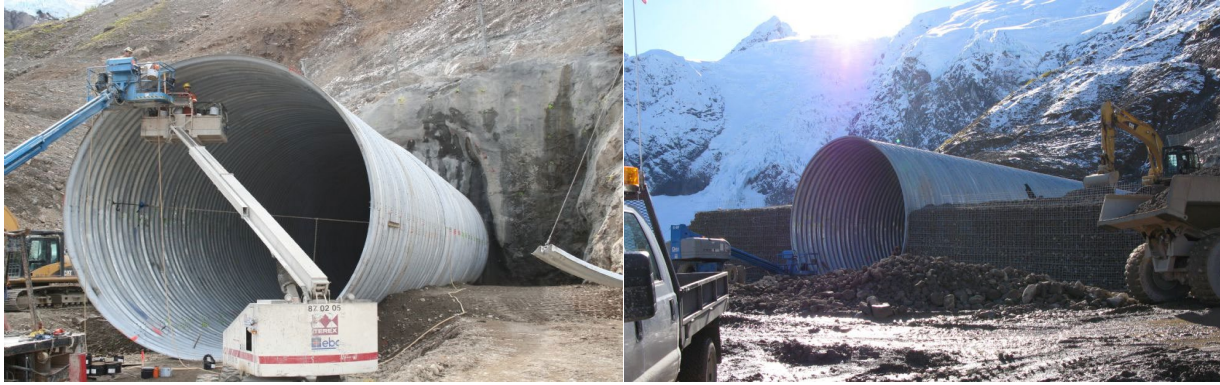
Figure 16: Installation of the multi-plate structure at Galore Creek Mine access road North Portal canopy after excavation and site preparation (left) and during completion of the backfilling (right). Photos: D. Brox.
