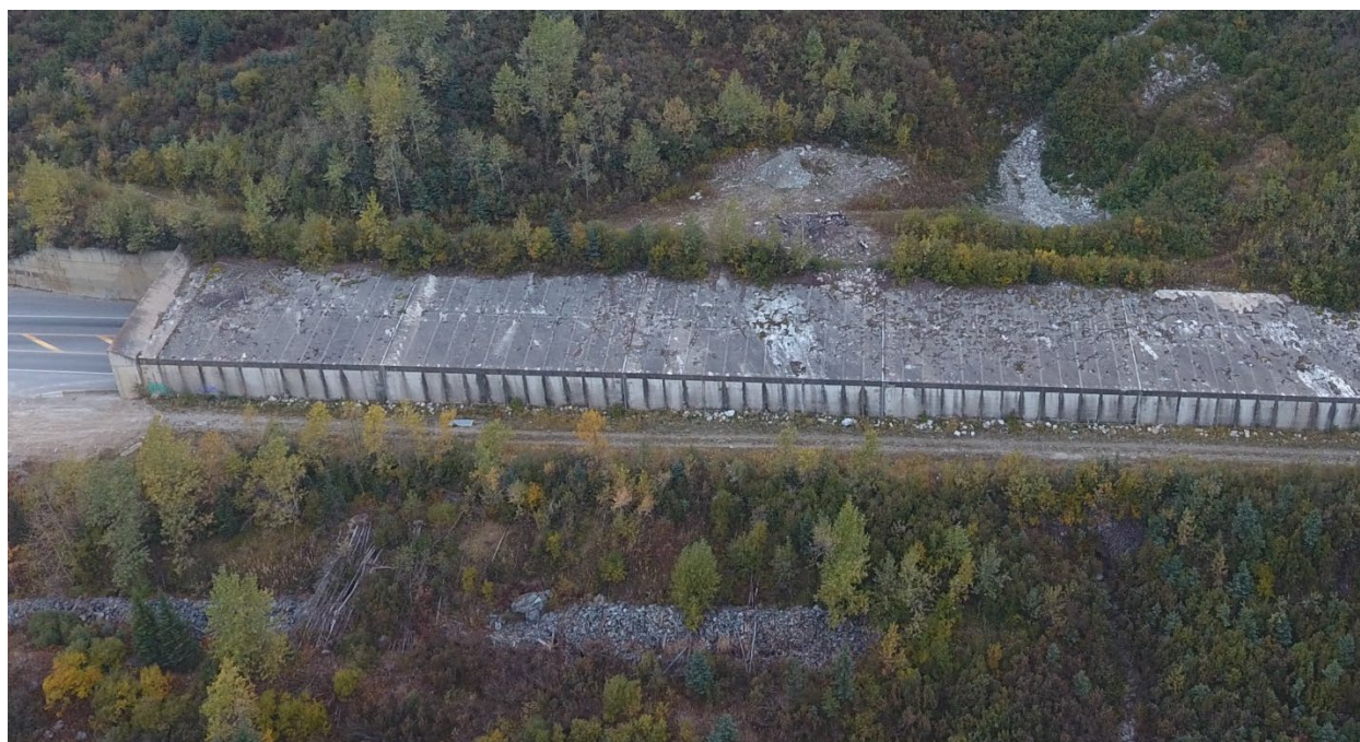
Figure 36: Single Bench snow shed in Rogers Pass, BC showing evidence of debris and rockfall impacts on the concrete roof slabs (Photo: Dynamic Avalanche Consulting)
