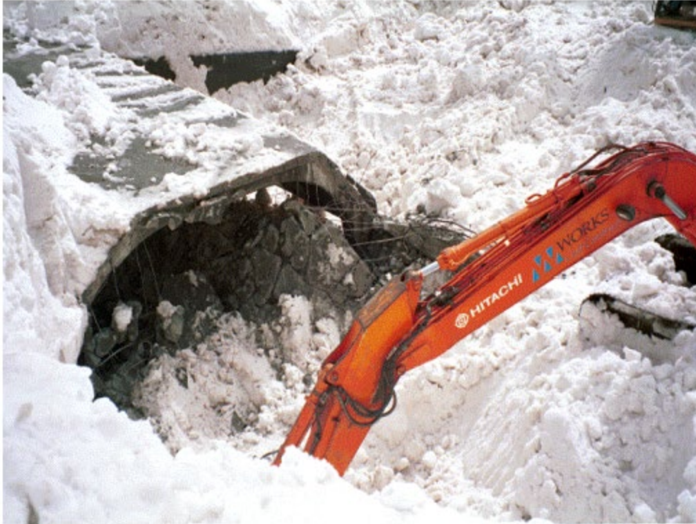
Figure 28: An avalanche on October 7, 1996 damaged the east portal of Homer tunnel. Impact pressures of 650-700 kPa were estimated, and resulted in damage to the reinforced-concrete portal structure (Conway et al., 2000).
