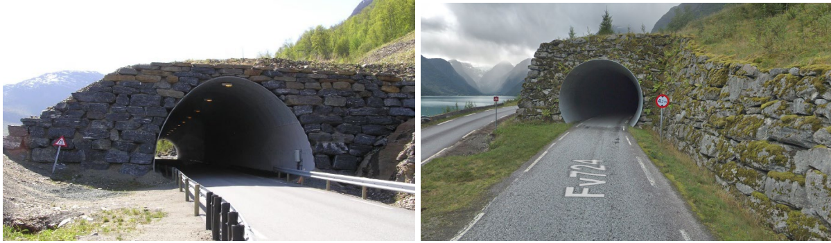
Figure 24: A snow shed near Ellevoll, in Troms, Norway (left) and in Olden, Vestland as examples of a CMP snow shed design. Photo from Tore Humstad and Google Maps, 2020 17 .
