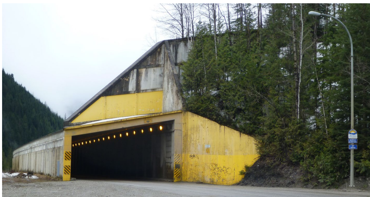
Figure 11: The cantilevered wing walls on the Lanark snow shed were constructed after the construction of the snow shed. The structures of the wing walls are independent from the shed structure and the additional load from the walls does not affect the snow shed (Photo: Alan Jones).
