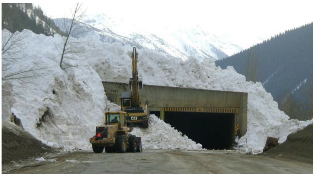
Figure 41: Single Bench overflow at the west portal due to a glide slab avalanche from the adjacent Mounds avalanche path, April 10, 2012. (Photo: Parks Canada Agency)
