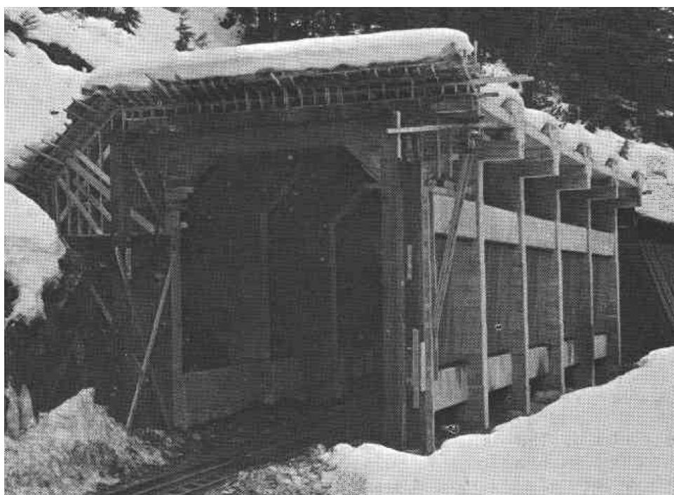
Figure 13: Snow shed in concrete at the Canadian Pacific Railway, built in 1960 (Photo: Schaerer, 1967)
