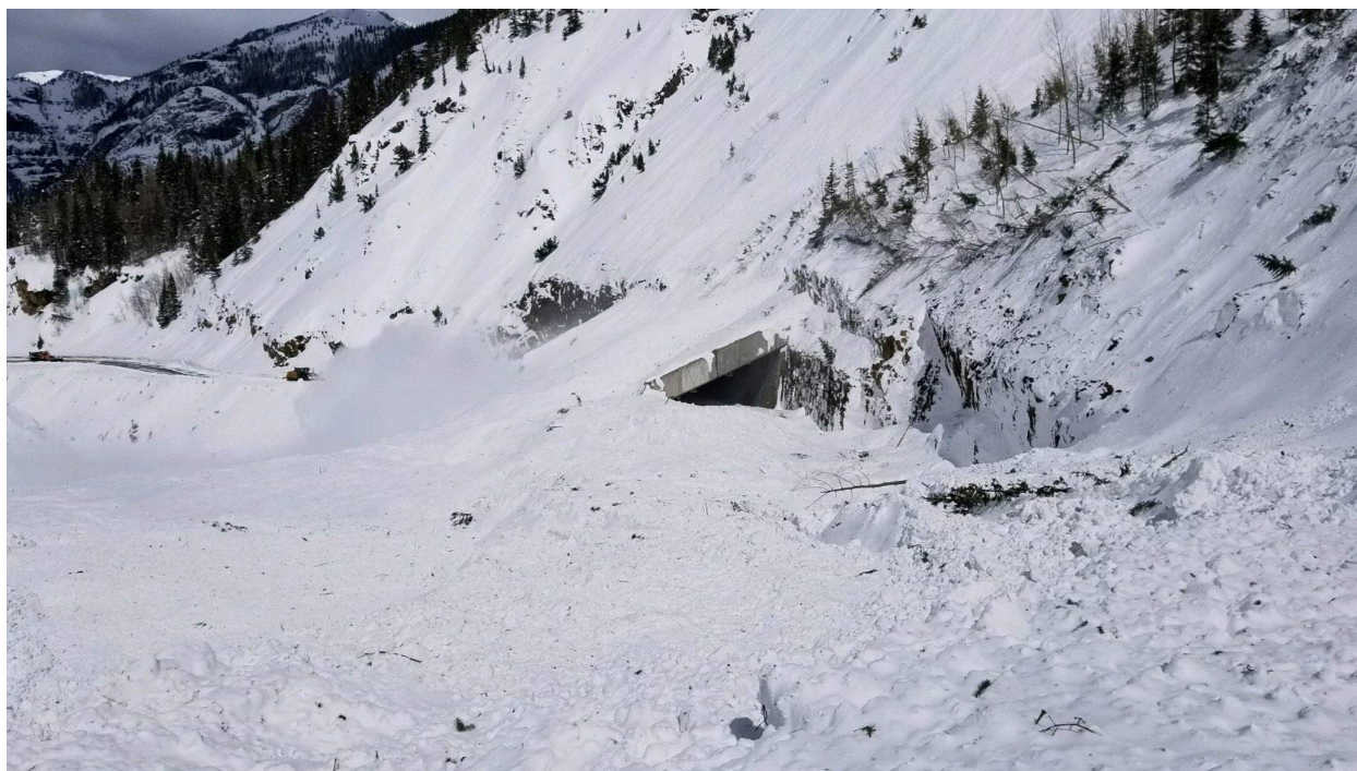
Figure 4: The Riverside snow shed covered in avalanche debris following mitigation work by the Colorado Department of Transportation. March, 2019 (Photo: CDOT).
