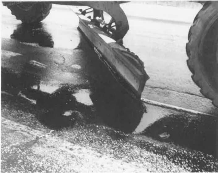
Photograph No. 3 Squeegee Seal
