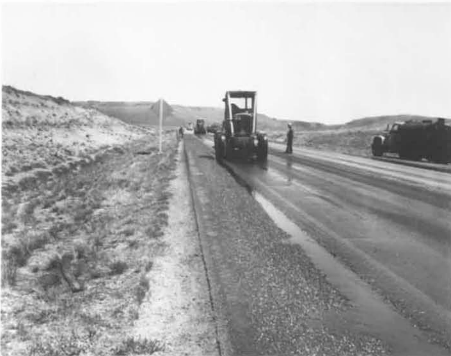
Photograph No. 4 Squeegee Seal
