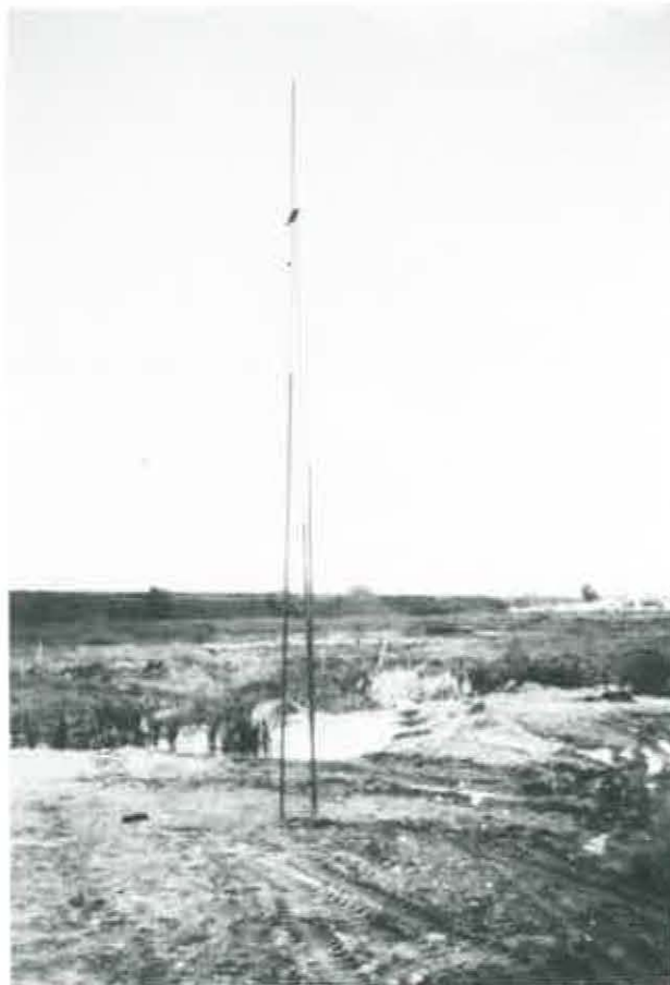
FIGURE 19. FINAL VIEW OF THREE ANCHORS INSTALLED IN TEST SECTION NO. 1. THE INNER TUBES WERE MONITORED FOR SUBSURFACE GROUND MOVEMENTS
