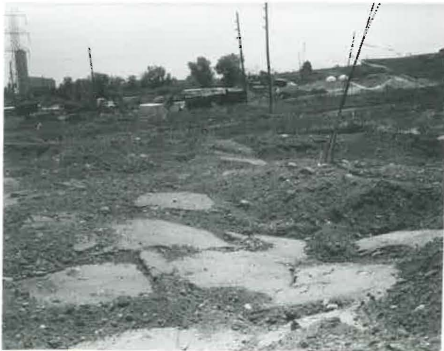
FIGURE 26. VIEW OF TEST SECTION NO. 1 AT THE END OF THE IRONING PHASE
