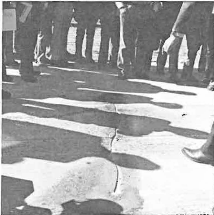
The routed crack is inspected by a group of attendees just prior to cleaning and sealing. Sealing the cracks and joints is the last activity in the complete CPR system.
