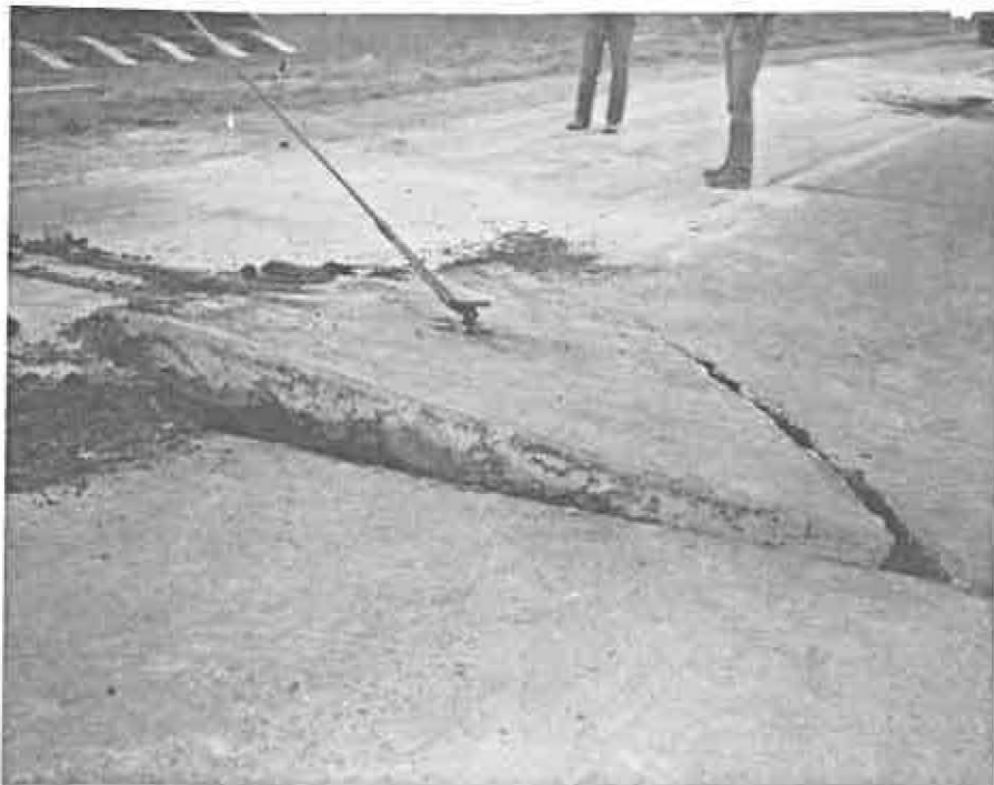
Removal and placing of old, broken concrete slabs is the first CPR procedure. Pictured is an 8 inch slab being lifted out of place. Prior to removal the slab was outlined with a full depth sawcut. Eight inch concrete will replace the old removed slab.
