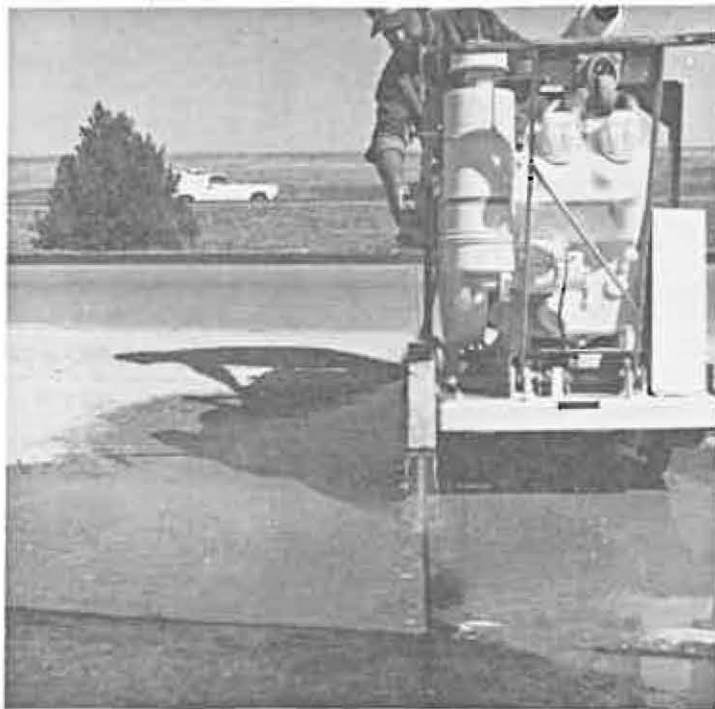
The last CPR procedure that the contractors demonstrated was the resealing of joints and cracks. Here, a diamond saw is refacing a concrete transverse joint.
