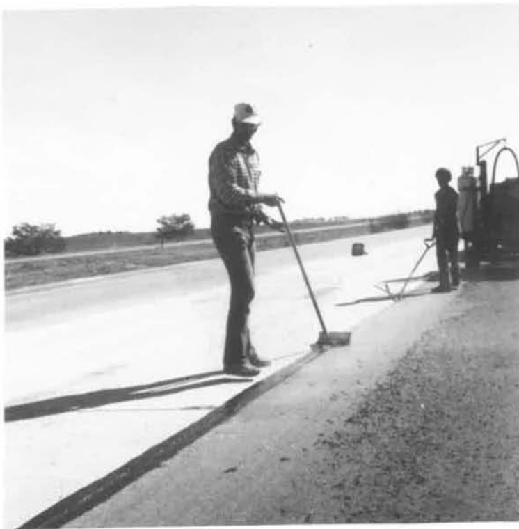
Hot rubber - asphalts are placed with a heated pressurized wand and squeegeed to level with the surface.
