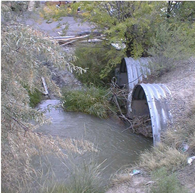
Figure 5. Example of Common Maintenance Need
