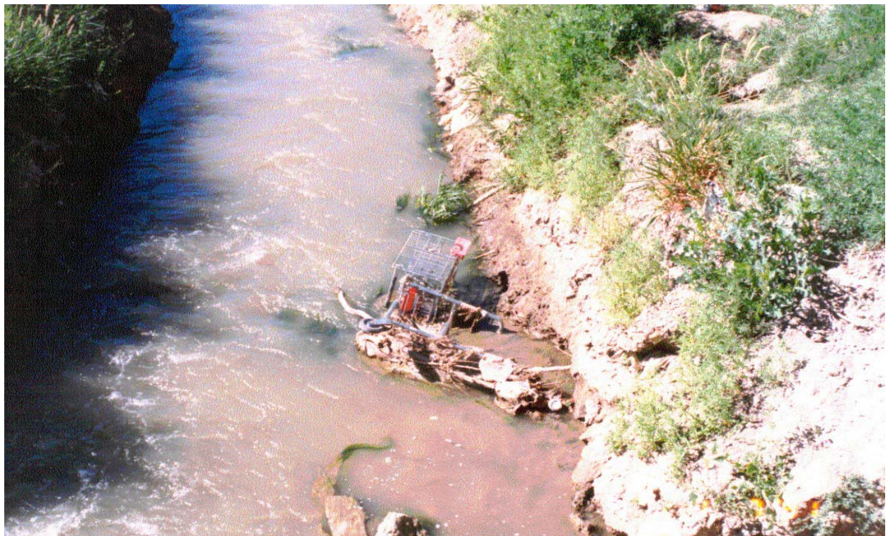
Figure 4. Example of Common Maintenance Needs
