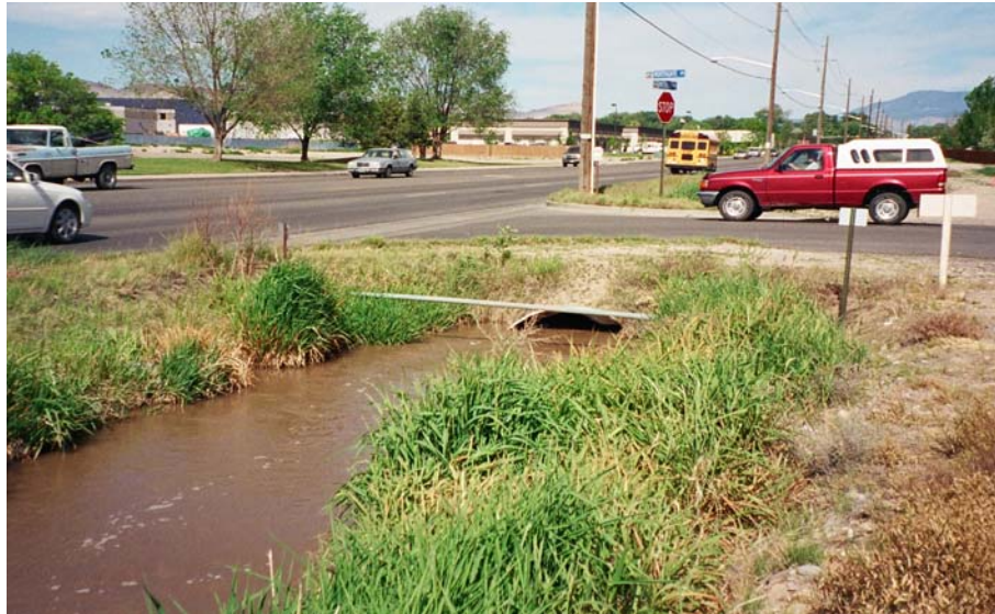
Figure 13. Horizon Drive Channel Shown Flowing Full of Irrigation Water Patterson Road at N. Westgate Avenue, May 2003 (Limited availability for storm water)
