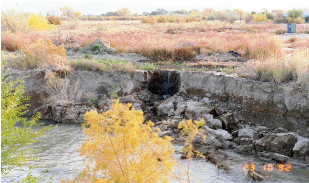
Figure 11. Bank Erosion in Leach Creek just North of F ¼ Road (North of Mesa Mall)
