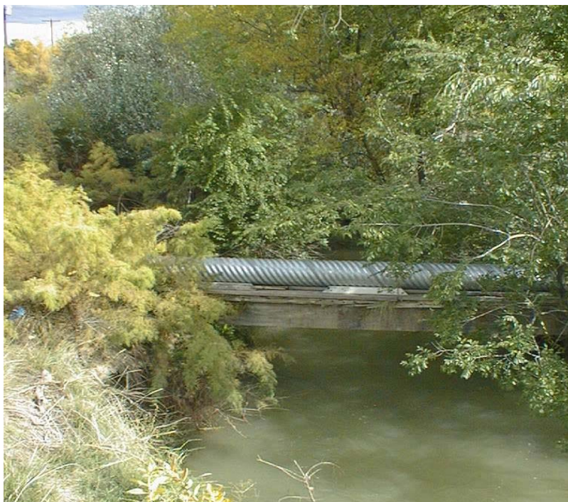
Figure 6. Utility Crossing and Overgrown Channel
