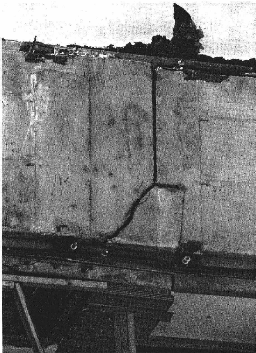
Swelling soil damaged the Life Sciences Building at the Southern Colorado State College campus near Pueblo.
