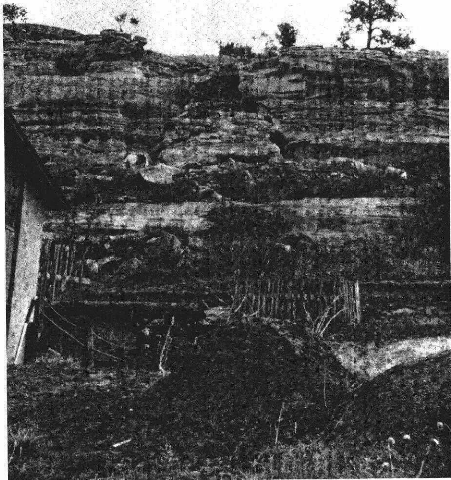
A typical rockfall hazard area on the steep west side of a hogback south of Denver. The massive sandstone blocks exposed at the top of the hogback can roll to the base of the hogback.
