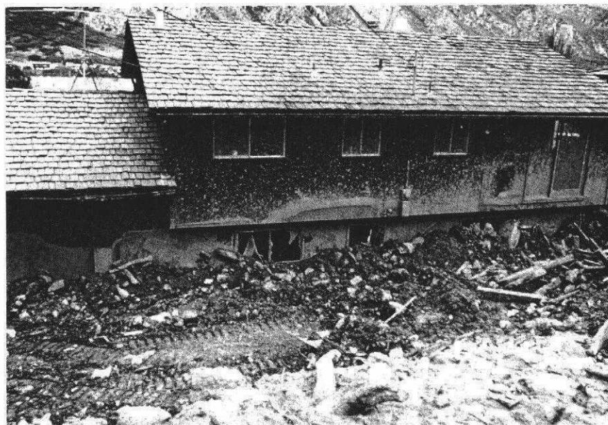
A debris flow smashed into this Glenwood Springs home in 1977. The house is a part of a residential development placed on a debris fan which had been built up over the years. Note the height of the flow as indicated by the water/mud mark at second floor level.
