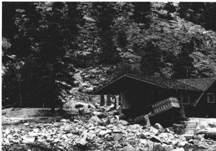
This house was located on a debris fan of a small tributary to the Big Thompson River. The house was not damaged by mainstream flooding on the Big Thompson, but by the debris flow from the small ravine behind the house.
