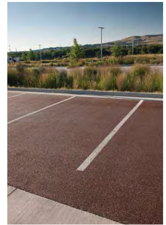
Permeable paving can be successfully installed in low-traffic areas including parking stalls and plazas.
