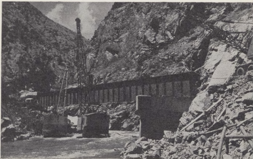
Road building up the narrow Cañon required that cranes wade in the creek.
