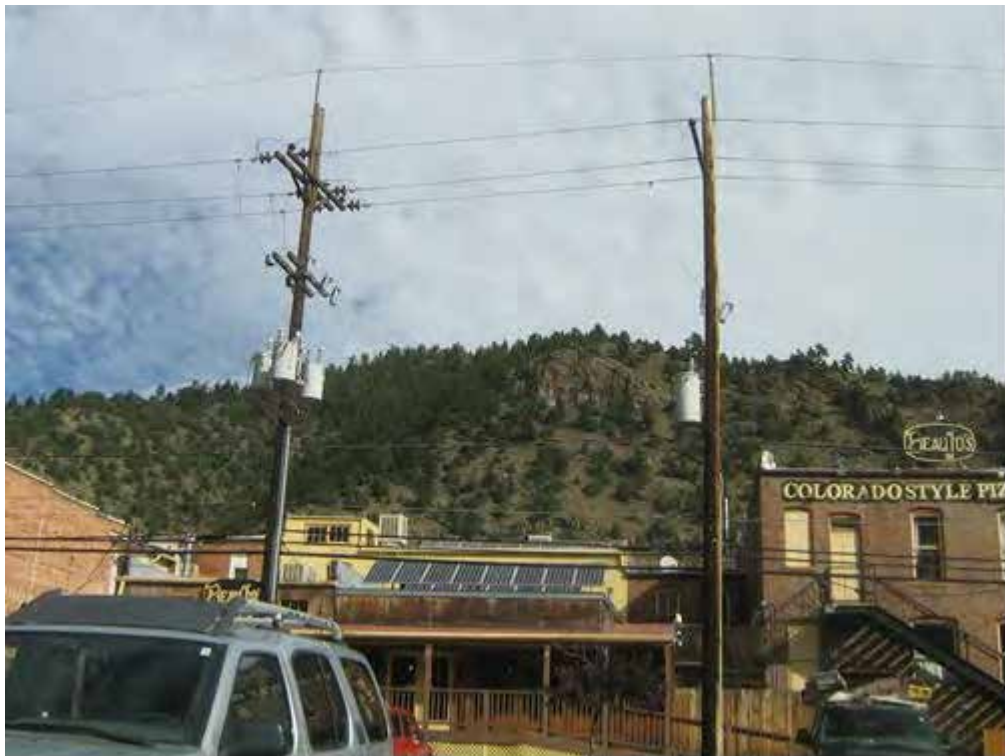
Photo 4. View of typical pole mounted transformers found throughout the project vicinity. No pole mounted transformers were found on the Site.
