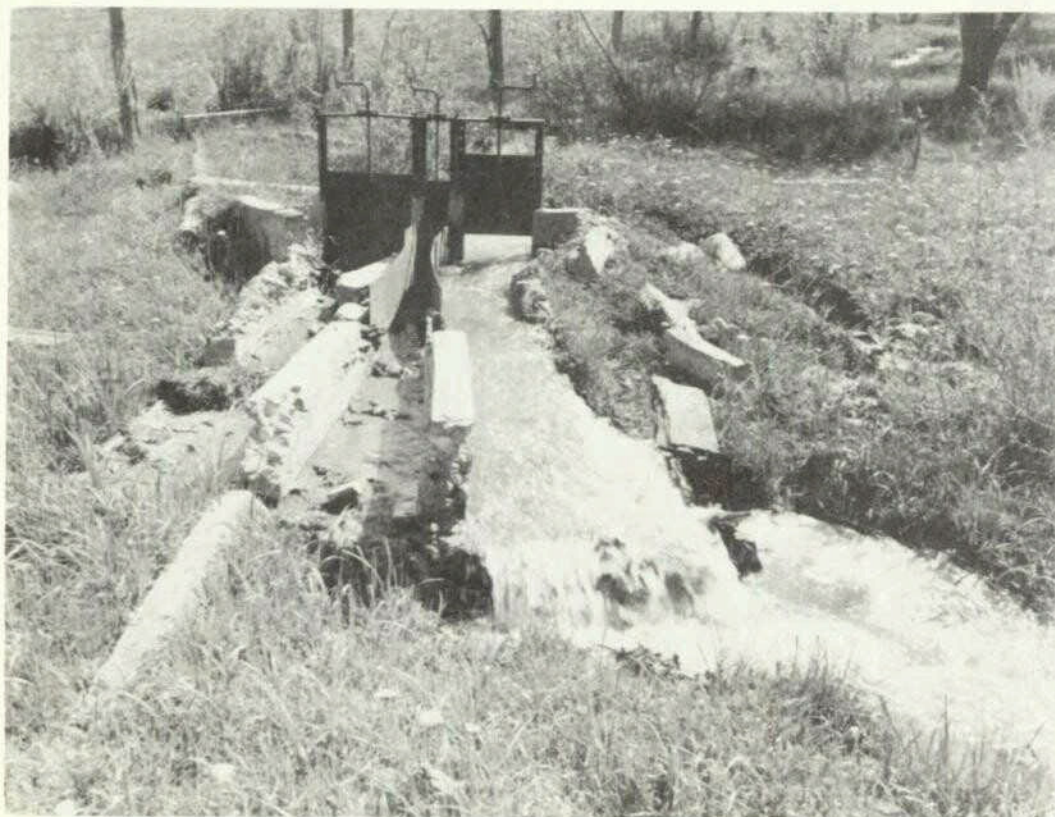
Mancos Valley - Water control structures need to be replaced
