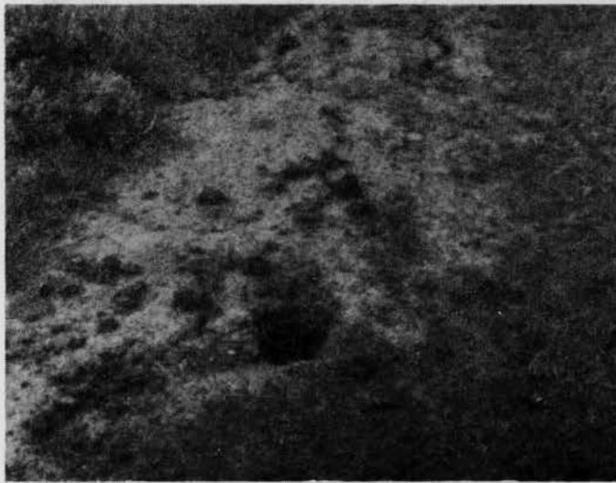
PHOTO 7.5-5 — RODENT HOLE FOUND ON THE CREST OF A DAM
