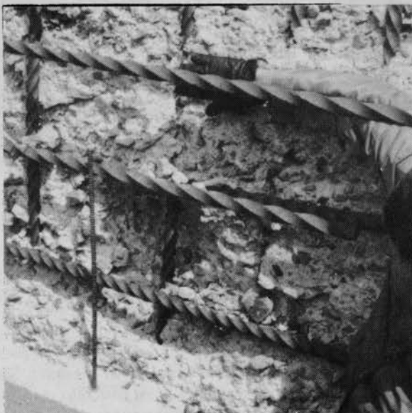
PHOTO 11.4-3 — STRUCTURAL DAMAGE. Spalling has exposed reinforcing.
