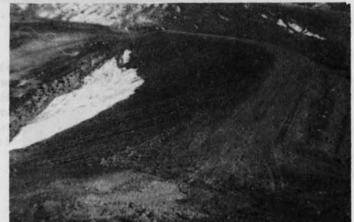
PHOTO 7.5-9 — CAMBER INCORPORATED INTO CREST DURING CONSTRUCTION. Camber is greatest over highest section of the dam.
