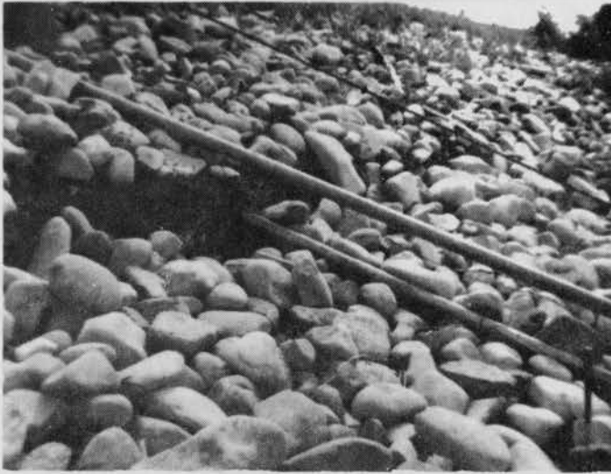
PHOTO 6.5-1 — UNIFORM POORLY SIZED RIPRAP LEADS TO EROSION OF SOIL BEHIND RIPRAP.
