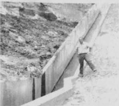
PHOTO 10.5-3 — WATER EXITING AT JOINT OR CRACK BECAUSE OF POOR DRAINAGE.
