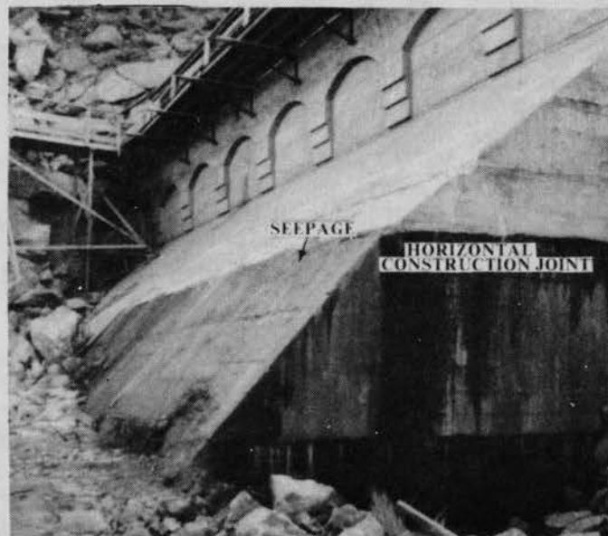
PHOTO 11.4-2 CRACKS AT HORIZONTAL CONSTRUCTION JOINT. Note evidence of minor leakage.
