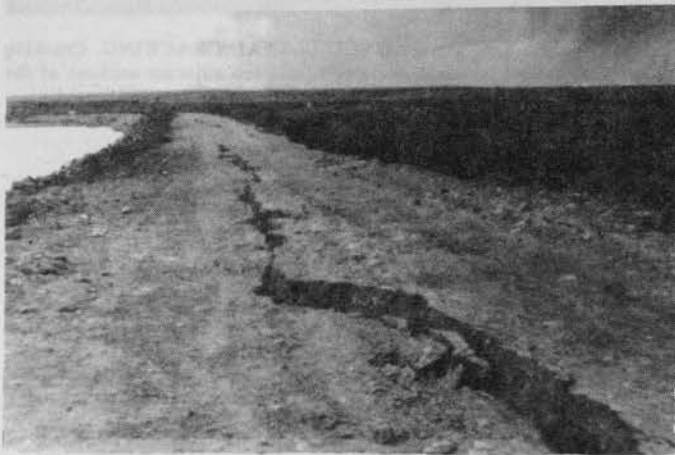
PHOTO 7.3-2 — VERTICAL DISPLACEMENT ON THE CREST OF A DAM. IN ITS INITIAL STAGES, THIS CONDITION WAS DETECTED AS A LONGITUDINAL CRACK.
