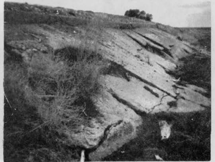
PHOTO 6.5-5 — BADLY DETERIORATED CONCRETE FACE
