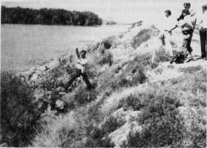
PHOTO 6.5-3 — CRACK IN UPSTREAM SLOPE
