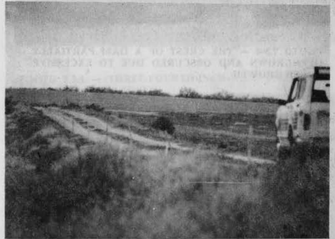
PHOTO 7.5-2 — LOW AREA IN THE CREST OF A DAM, CAUSED BY A FOUNDATION FAILURE.
