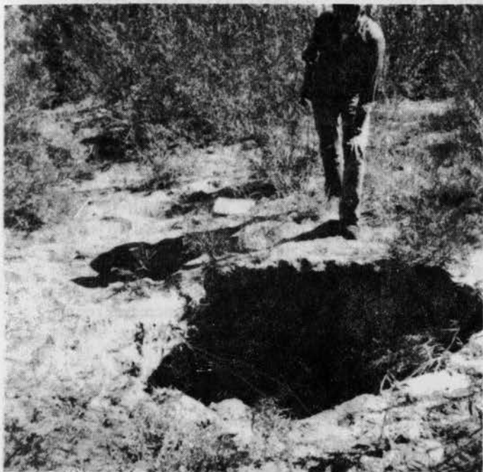
PHOTO 9.4-1 — SINKHOLE ON DOWNSTREAM SLOPE ABOVE OUTLET CONDUIT. Failure occurred as described in Figure 9.4-3.
