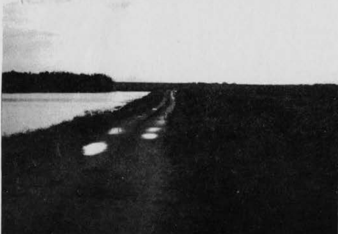
PHOTO 7.3-4 — CREST IN POOR CONDITION SHOWING EVIDENCE OF MISALIGNMENT.
