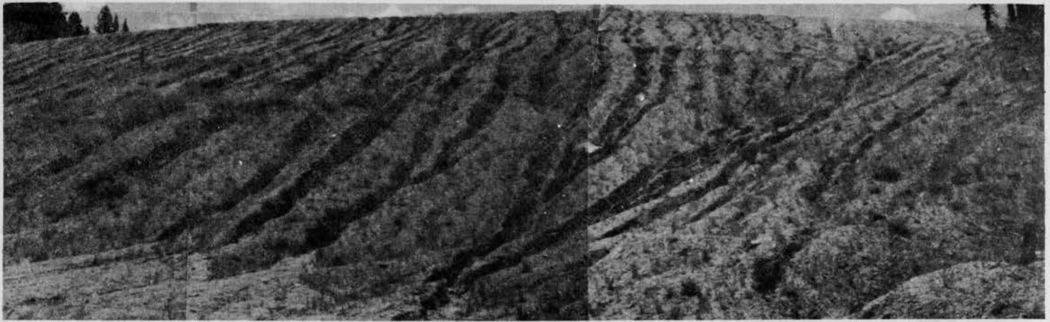
PHOTO 8.5-1 — EROSION D/S FACE
