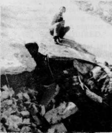
PHOTO 10.5-4 — FAILED SPILLWAY Fracturing of spillway chute slab
