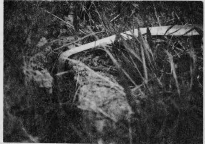
PHOTO 8.3-1 — THREE-FOURTH-INCH-WIDE CRACK, WELL HIDDEN IN GRASS COVER.
