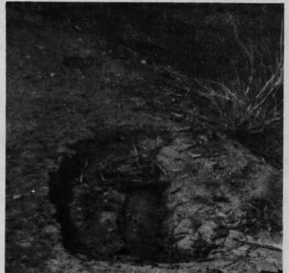
PHOTO 7.5-3 — SINKHOLES IN THE CREST OF A DAM, CAUSED BY CONSOLIDATION OF LOW DENSITY EMBANKMENT MATERIAL.
