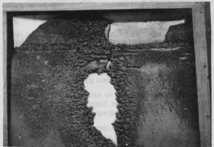
PHOTO 9.3-2 — CAVITATION DAMAGE TO STEEL PIPE LINER. Cavitation has eaten through steel to expose concrete behind liner.
