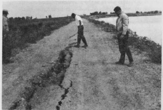
PHOTO 7.3-1 — SEVERE LONGITUDINAL CRACKING. Cracking pattern indicates horizontal movement between adjacent sections of the dam. Note the close parallel cracks.
