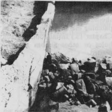
PHOTO 10.5-1 — DETERIORATION OF RIGHT D/S WINGWALL OF SPILLWAY.
