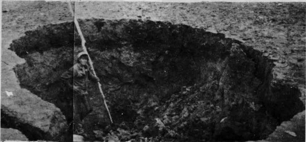
PHOTO 6.5-8 — 21' x 21' SINK HOLE IN RESERVOIR BASIN
