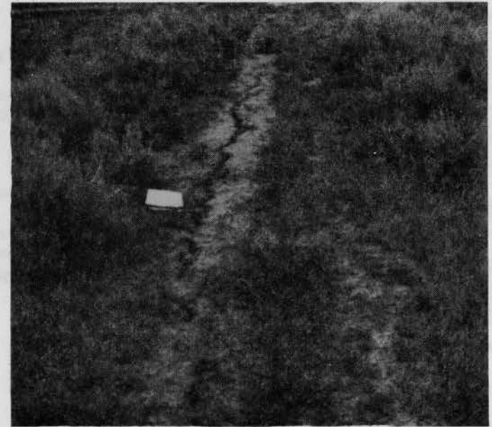
PHOTO 7.5-8 — LONGITUDINAL DRYING CRACKS ON THE CREST OF A DAM. These cracks are caused by drying of the crest surface and are only 6-8 inches deep.
