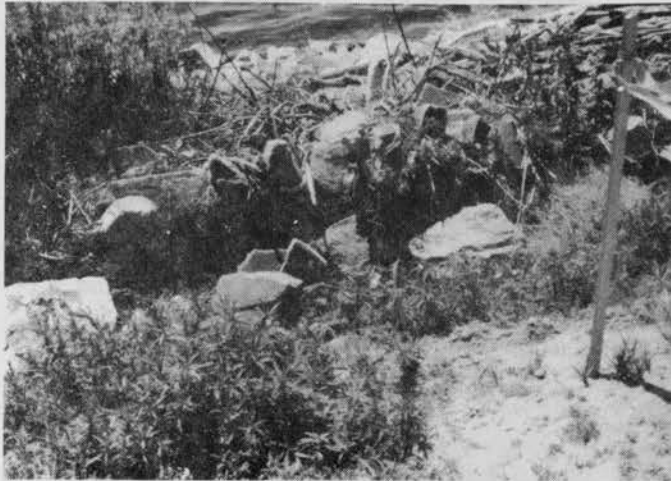
PHOTO 6.5-2 — CRACK IN UPSTREAM SLOPE
