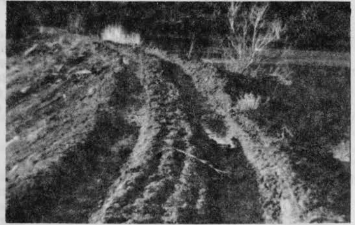
PHOTO 7.5-7 — RUTS IN THE CREST OF A DAM
