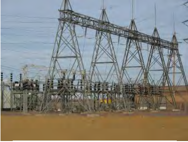
An Xcel electric substation in the corridor (East of Havana Street)
