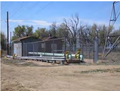
An Xcel gas utility station in the corridor
