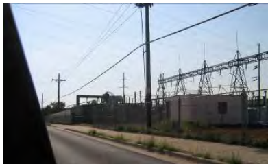
Electric utility station, high voltage utility poles with multiple lines. Looking southeast
