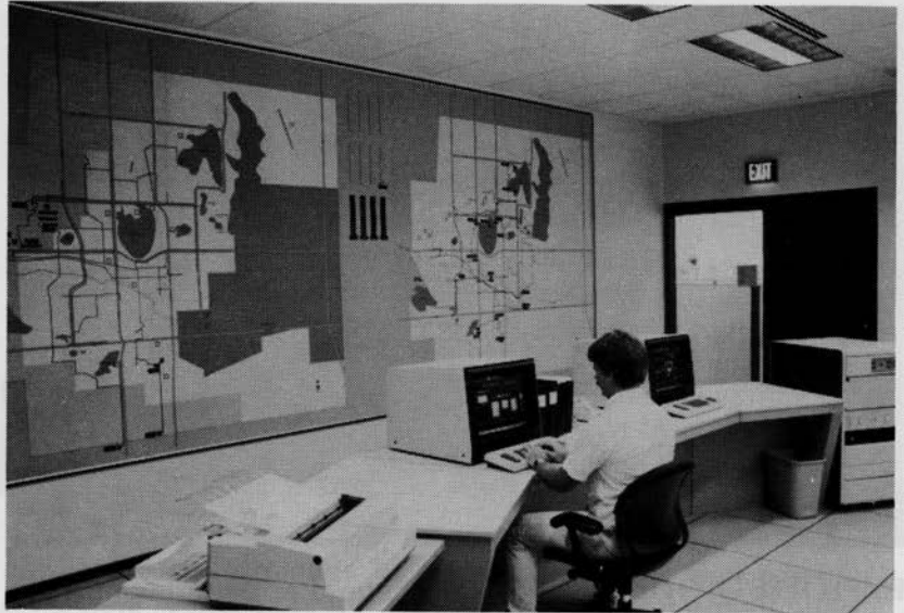
Tom Greene at the SCADA computer
