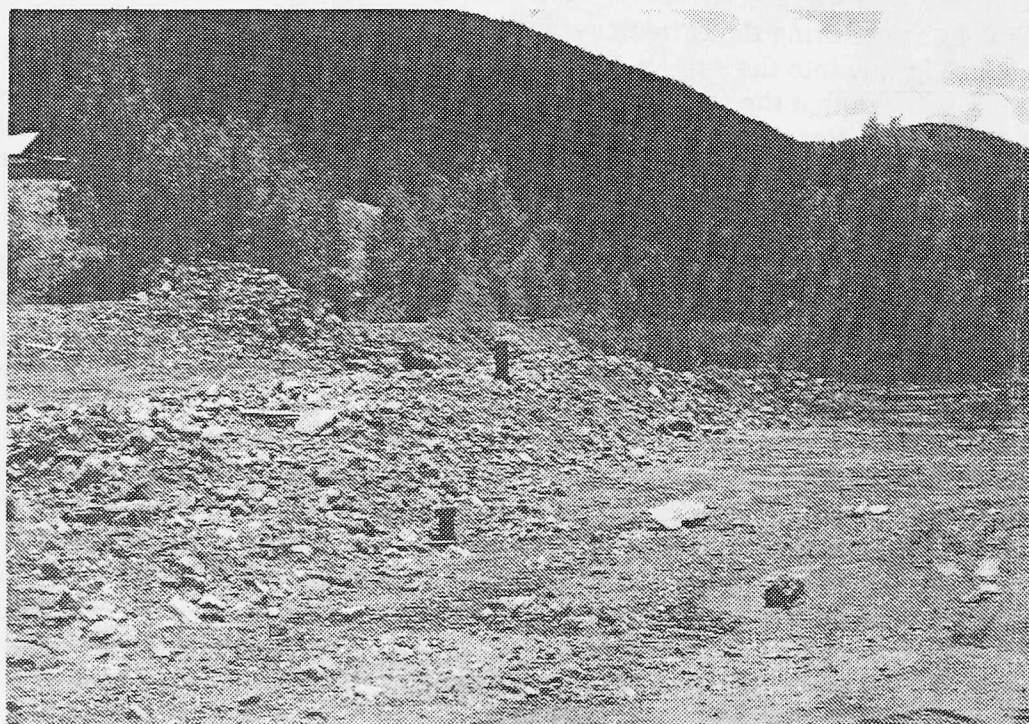
Figure 6. Water line on flooded bench. The riser pipe in the lower foreground and the hydrant are connected to the water line.
