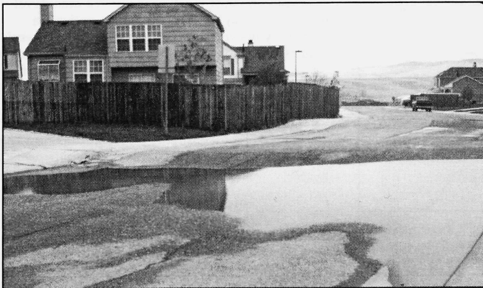
Figure 1. Linear heave feature associated with heaving bedrock in Douglas County. This heave feature has literally formed a dam that blocks storm drainage, resulting in surface-water ponding. Heaving bedrock has caused extensive damage in this neighborhood.
