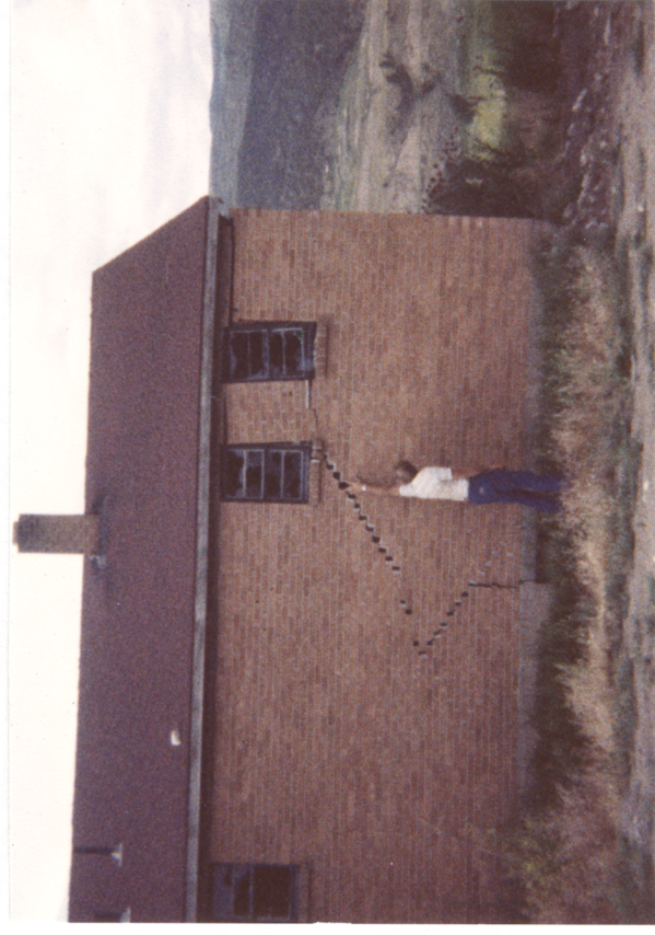
Soluble minerals in the Eagle Valley Evaporite formation are dissolved by groundwater. The resulting void sometimes causes subsidence at the surface. Subsidence (sink hole) resulted in this damage to a structure in Edwards, Colorado.
