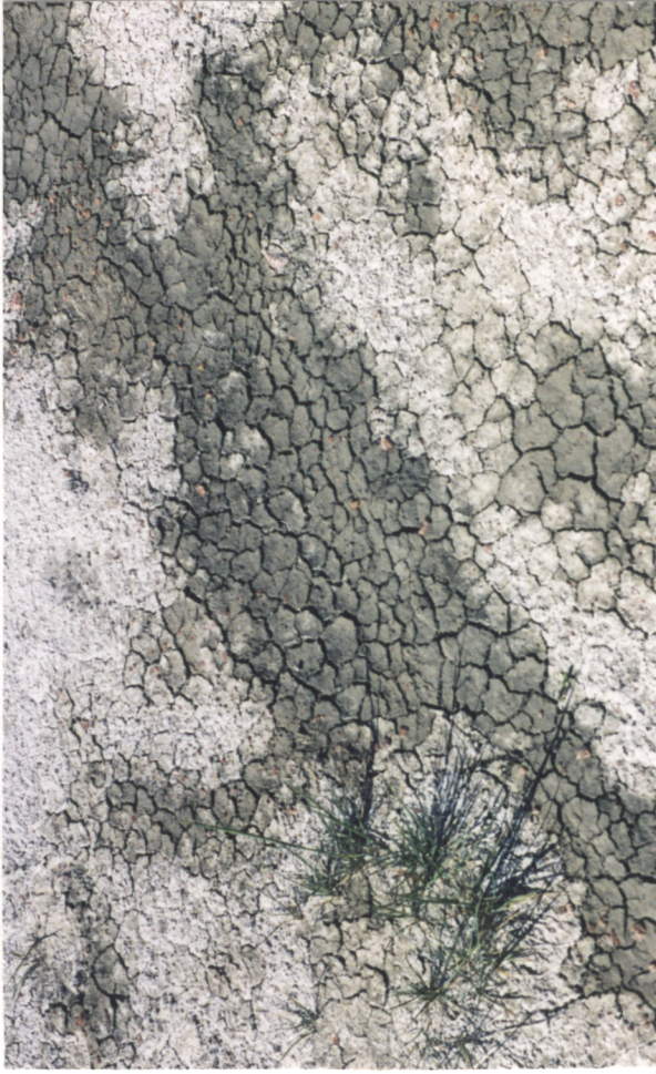
Shrinkage cracks form in expansive soils. Sulfate salts which are detrimental to concrete and metal leach out of corrosive soils.
