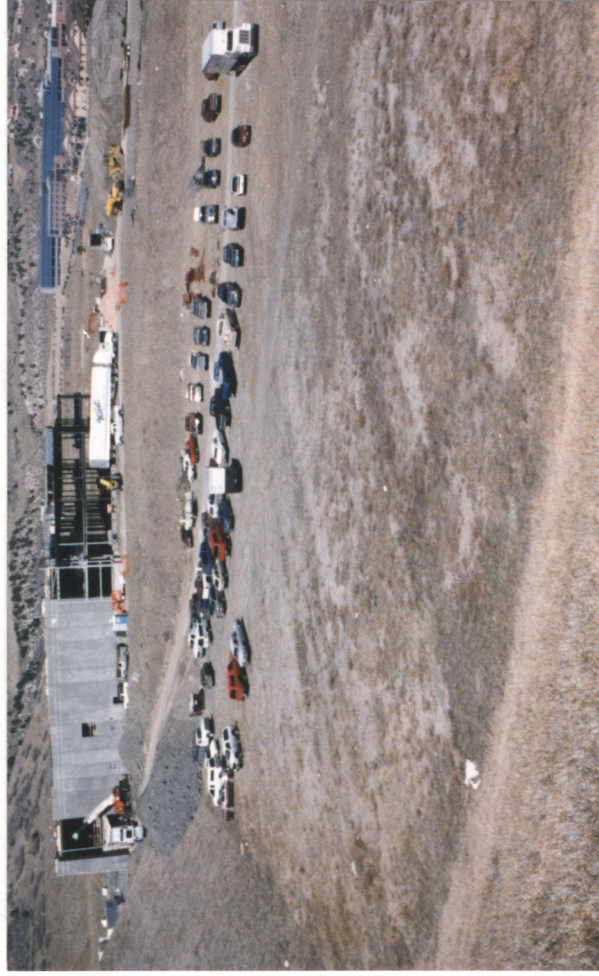
Several prominent linear heave features, which result from steeply dipping beds of expansive bedrock, cross a developed lot adjacent to an industrial development in Colorado Springs. All photos by John Himmelreich.
