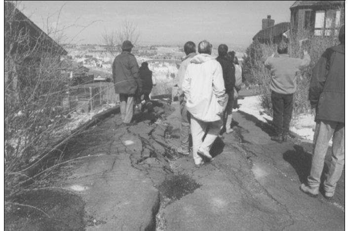
Landslide resulted in severe structural damage of two houses in Colorado Springs in 1995. Photos by John Himmelreich.
