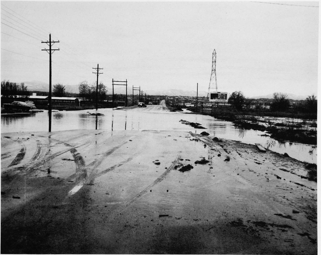
Figure 4. Flood damage on State Highway as result of thundershower in foothills region.
