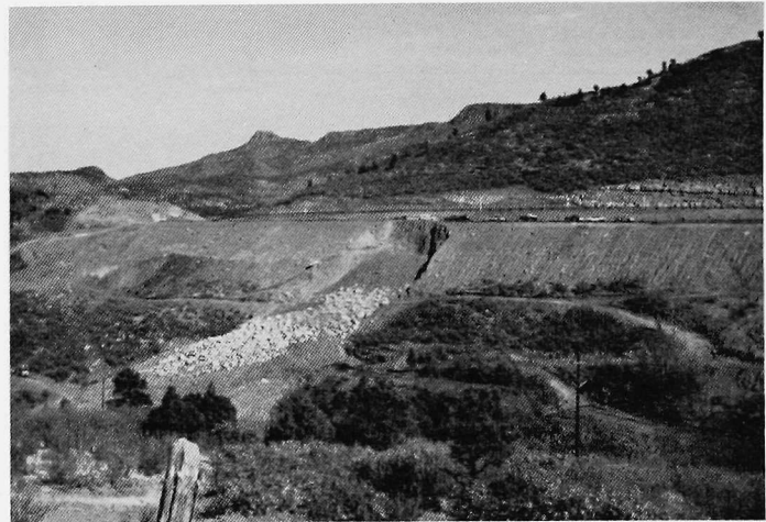
Figure 6. Failure of fill as a result of ground water.
