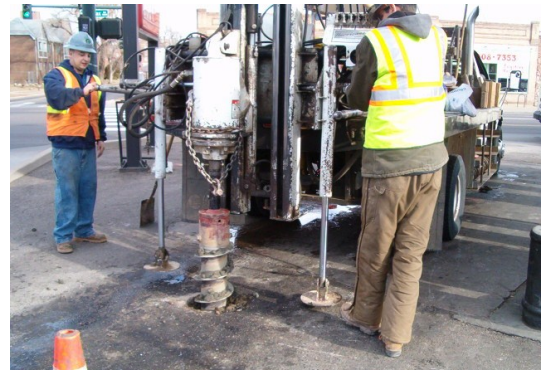
Hollow-stem auger drilling is an industry standard technique used to install groundwater monitoring wells.
