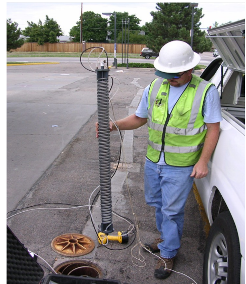
Supplying oxygen to contaminated groundwater accelerates remediation.
