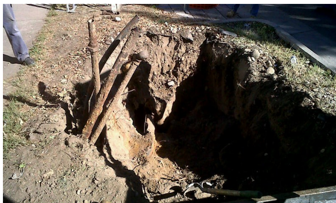
Tank removal excavation showing product piping that can be traced to former dispensing areas.
