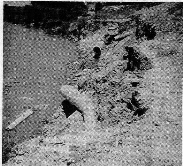
The Fountain Creek floodwaters washed out large sections of the embankment and a sanitary sewer trunk line. Photo courtesy of John Dagenais, City Public Works.
