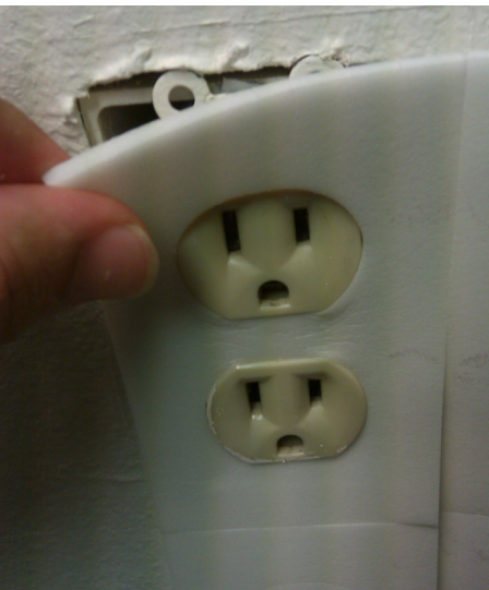
Figure 15. Foam gaskets are an easy fix to air infiltration from electrical outlets on exterior walls.
