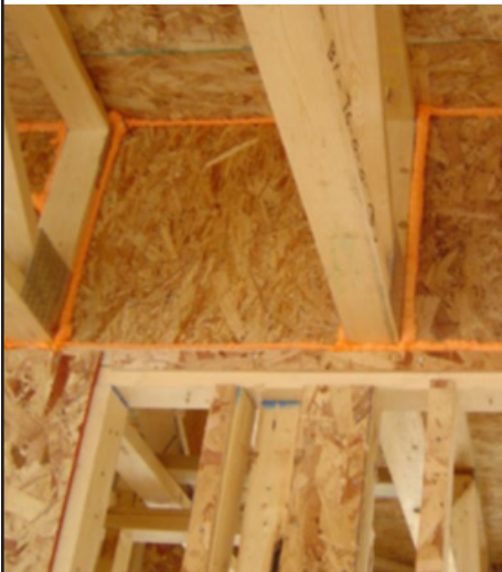
Figure 3. Joists running through a common wall of a garage can be sealed with caulk, spray foam, or water-based elastomeric sealant if exposed.
