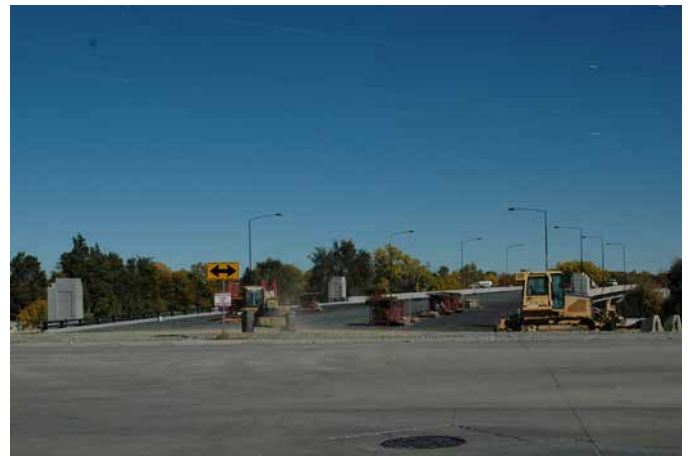
The 17th Place connection to I-225 (shown here under construction) will serve 35,500 vehicles per day.
