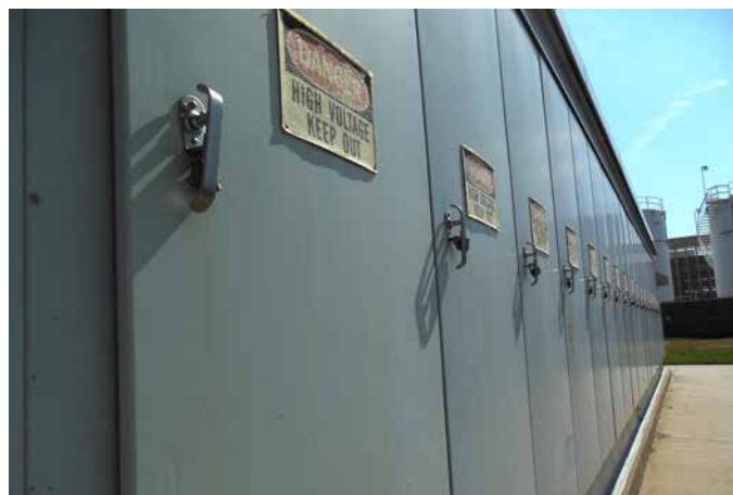
15kV main distribution outdoor switchgear.
