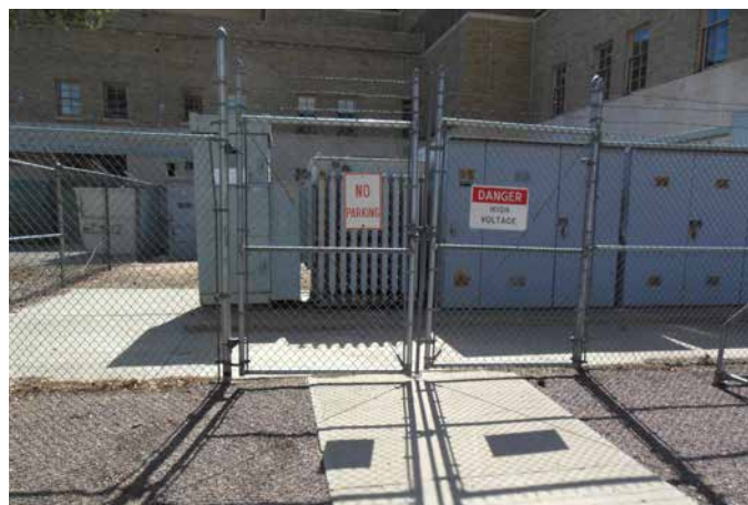
High-voltage area north of Building 500.
