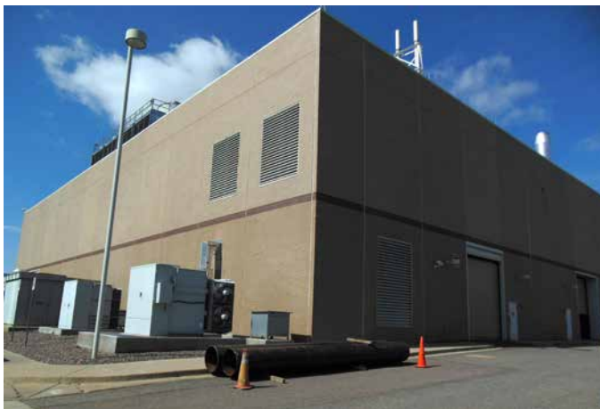
The CUP can accommodate boiler and generator expansions within the existing building envelope.
