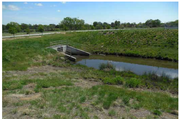
Water quality treatment infrastructure at Pond 374.
