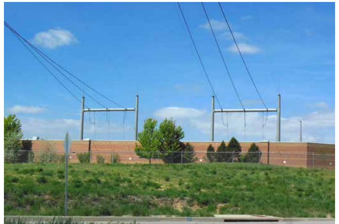
Xcel Energy Fitzsimons Substation.
