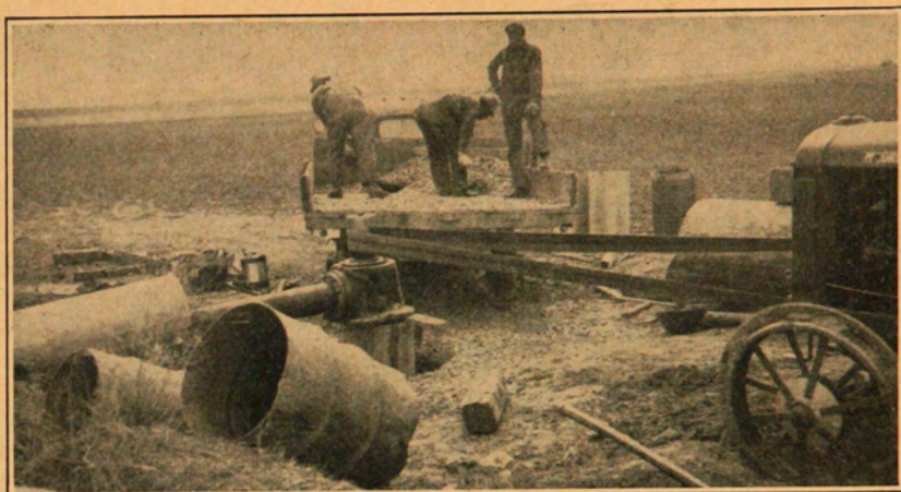
Figure 1.—Final stages of construction of an irrigation well. Applying gravel to outside of casing after removing larger outside blank casing and during test of well for capacity.
