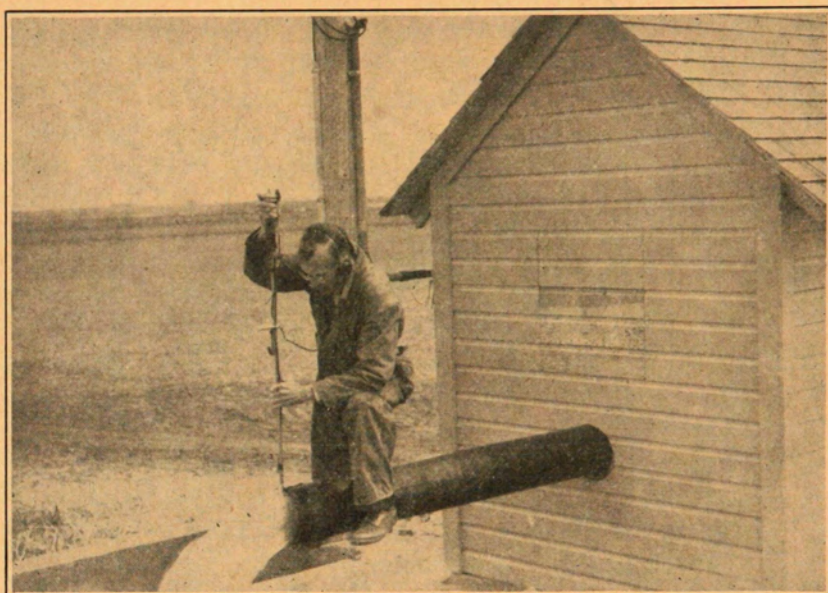
Figure 6.—Making discharge measurement with Hoff current meter. Pump is the turbine type in a shelter typical of the region.
