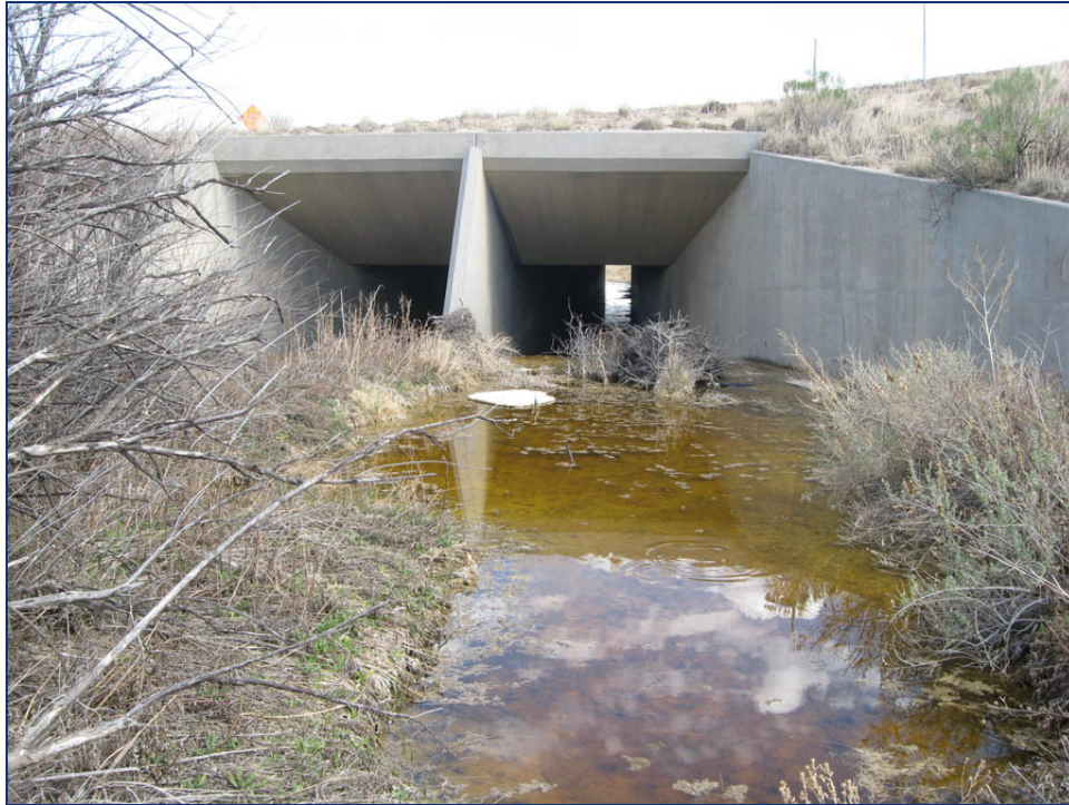
Figure H-3. Box Culvert and Ponding in Williams Creek Area EB US 50 at N. Pueblo Blvd.
