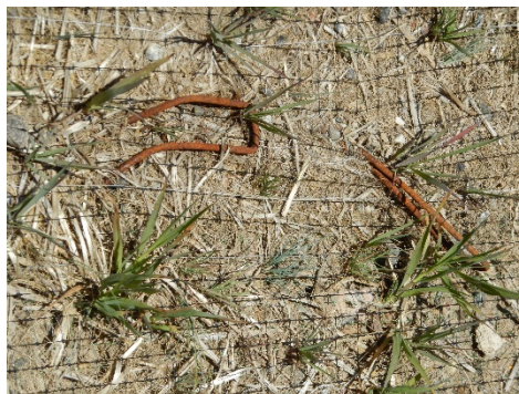
Picture 3. Blanket staples were not able to be installed completely likely due to soil compaction.
