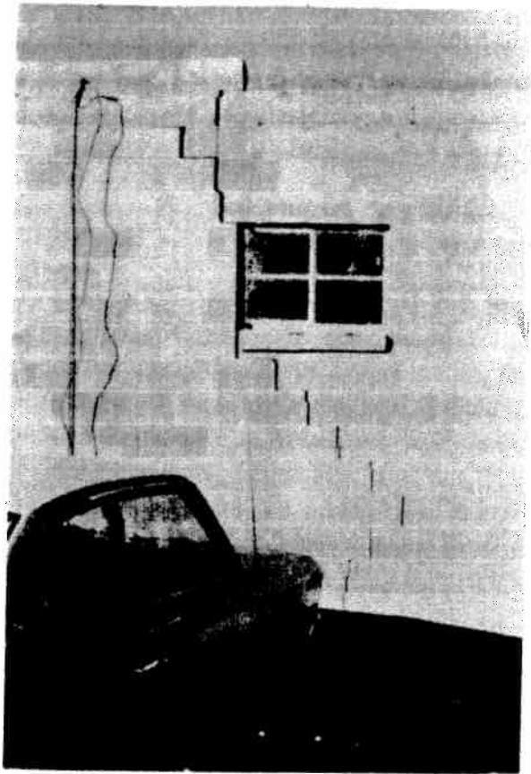
Figure 27. Damage to VFW hall, Main Street, Louisville. This part of Louisville was undermined many years ago. A seam 10 to 15 feet was extracted at a depth of about 100 feet. Because the mining occurred so long ago, it is thought that the damage to this relatively recent building is related to faulty design or construction, rather than to subsidence. Locality 43, subsidence-inventory map.
