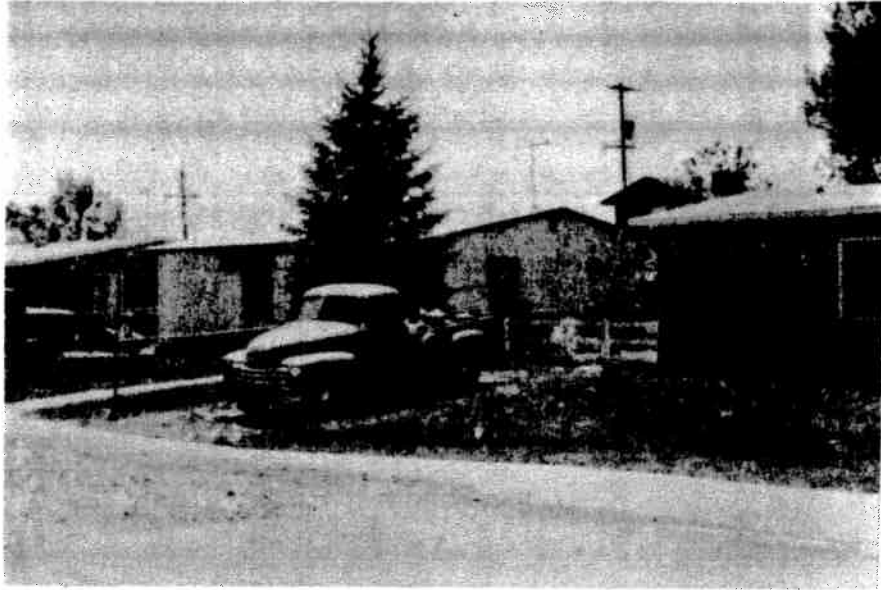
Figure 21. Subsidence over Strathmore mine, South Longmont Street, Lafayette. The most recent damage to the street has not yet been fully repaired. Note unpaved section of street and sagging sidewalk. The coal seam in this area of the Strathmore mine was quite thick, and the probable thickness of coal extracted was 20 to 25 feet. Depth of mining was 100 to 125 feet. Locality 55, subsidence-inventory map.
