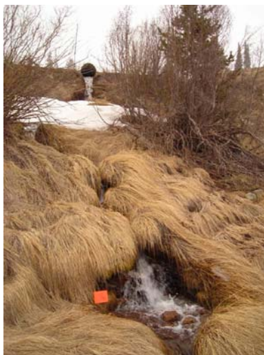
Figure 7. Unnamed tributary UT-3.212, the first and main iron fen tributary, followed a clear channel from the culvert under County Road 12 to Coal Creek; the sample was taken at the location of the orange flag within about 2 m of the creek’s north bank.
