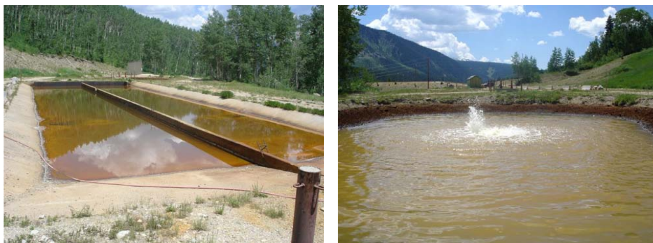
Figure 32. Photographs of the grit chamber (left) and equalization pond (right) used by the Mount Emmons treatment plant. The chamber and pond are located above the Keystone Mine drainage that forms part of unnamed tributary UT-5.368.
