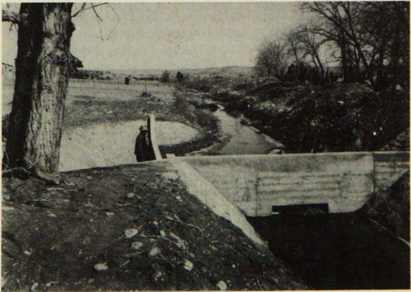
CARL HOLZMAN GATE REGULATES FLOW OF WATER IN DITCH. OLD DITCH USED FOR WASTE-WAY FOR FLOOD WATERS.
