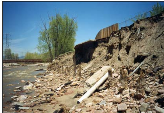
Figure 2-39. Flood damage on Fountain Creek Trail, Colorado Springs, 1999.
