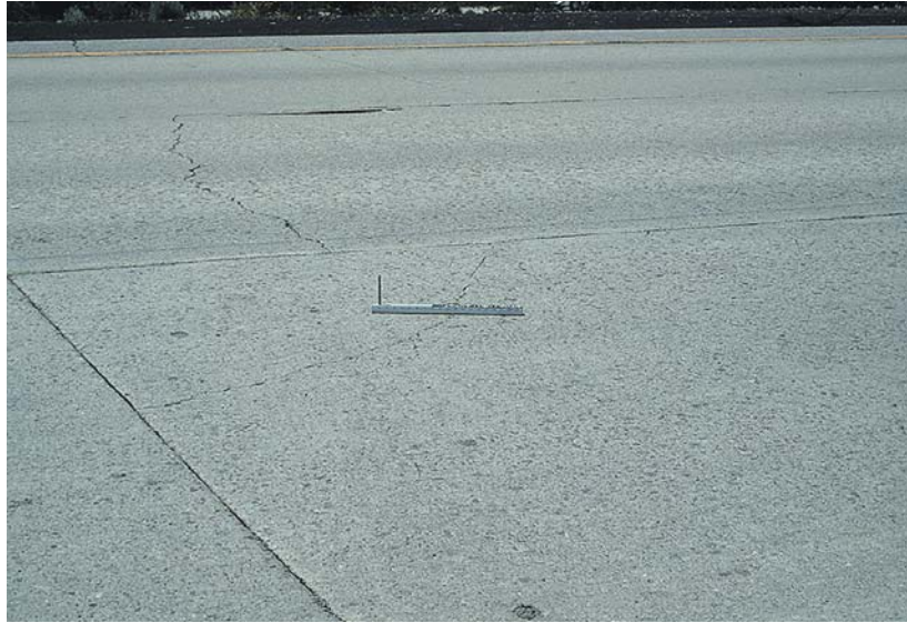
Figure 33 - Low Severity Corner Break
