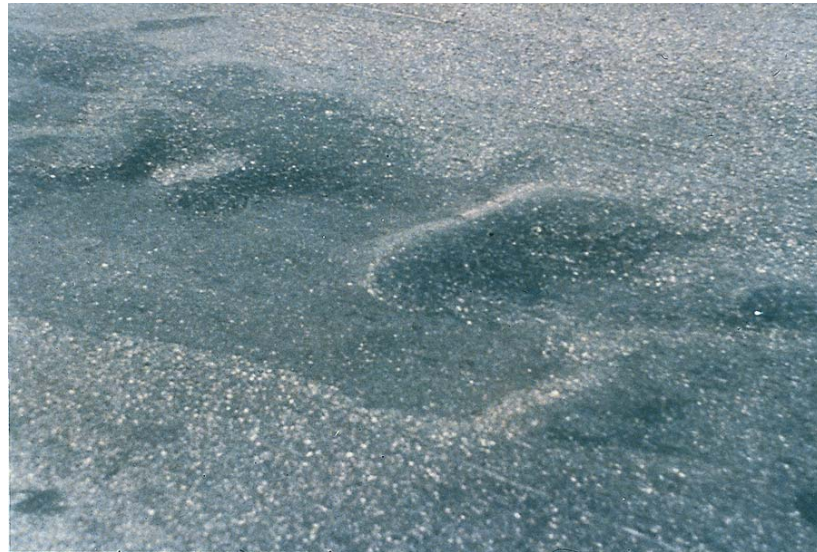
Figure 24 - Shoving in Pavement surface
