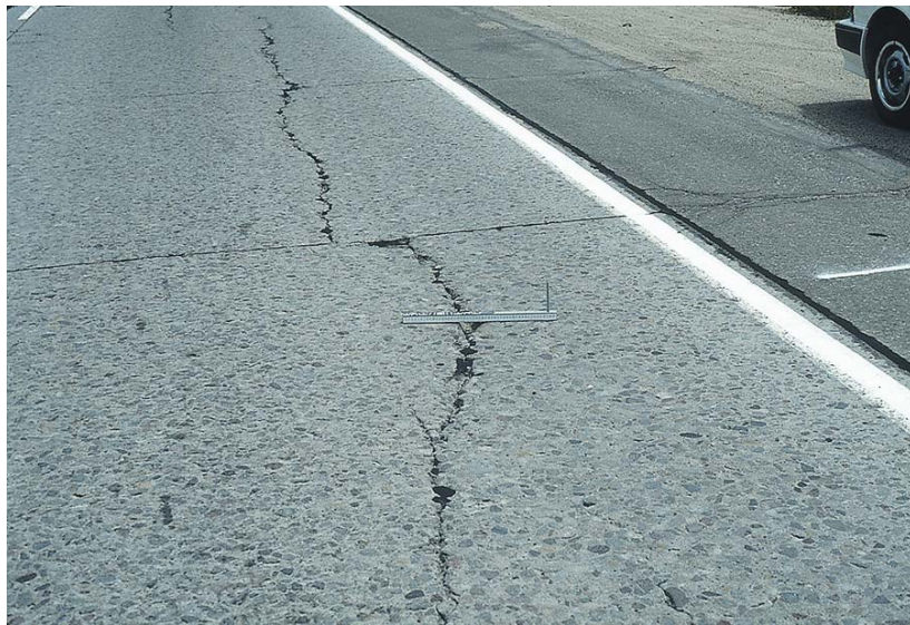
Figure 41 - High Severity Longitudinal Cracking
