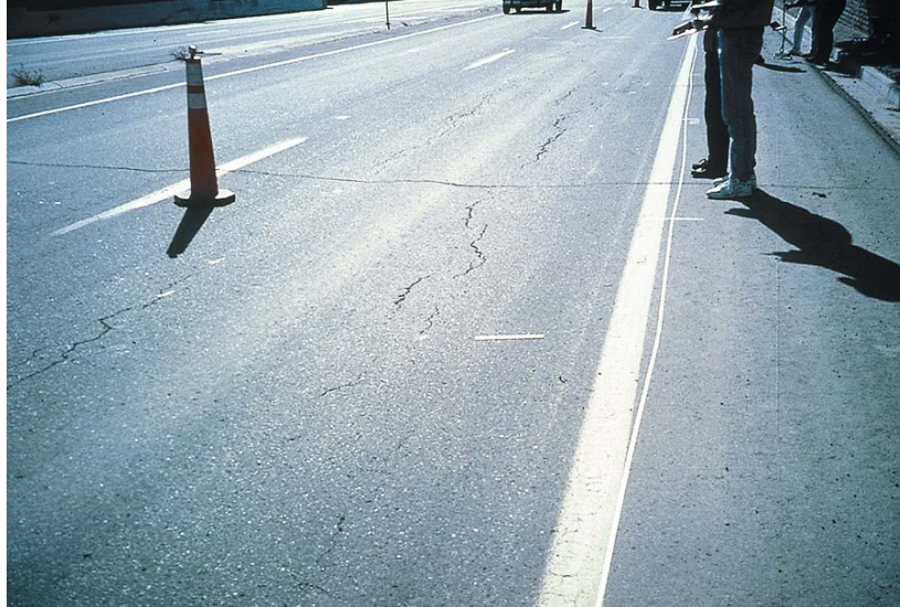
Figure 3 - Low Severity Fatigue Cracking
