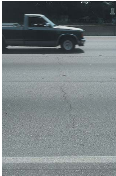
Figure 17 - Low Severity Transverse Cracking
