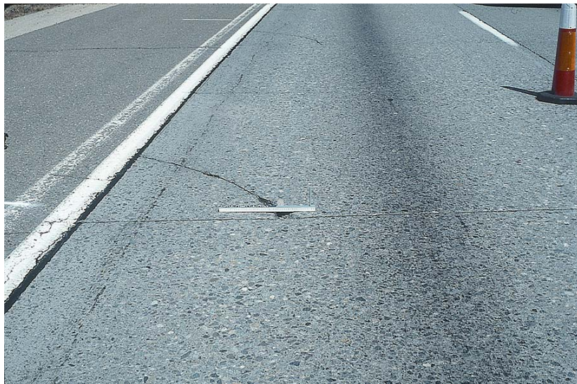
Figure 34 - Moderate Severity Corner Break
