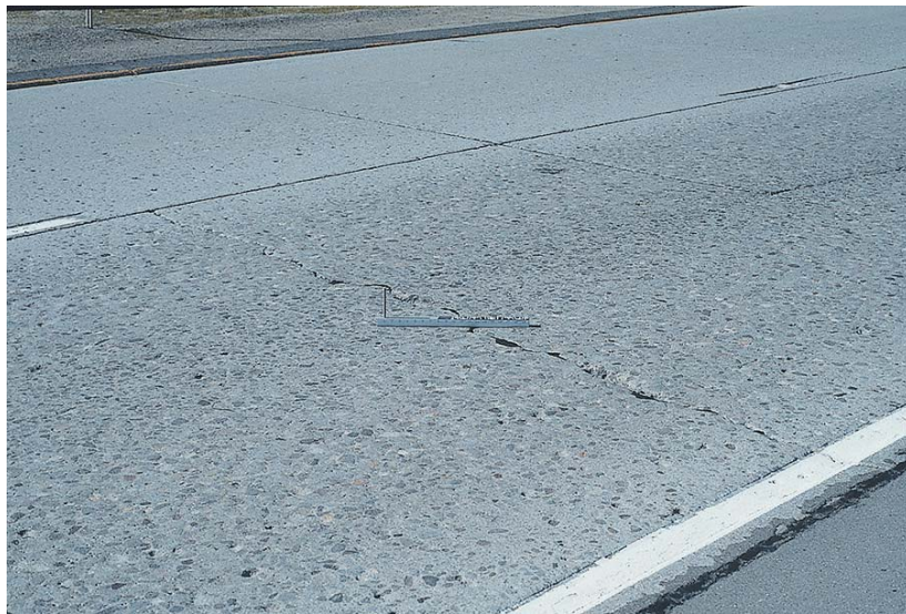
Figure 44 - High Severity Transverse Cracking
