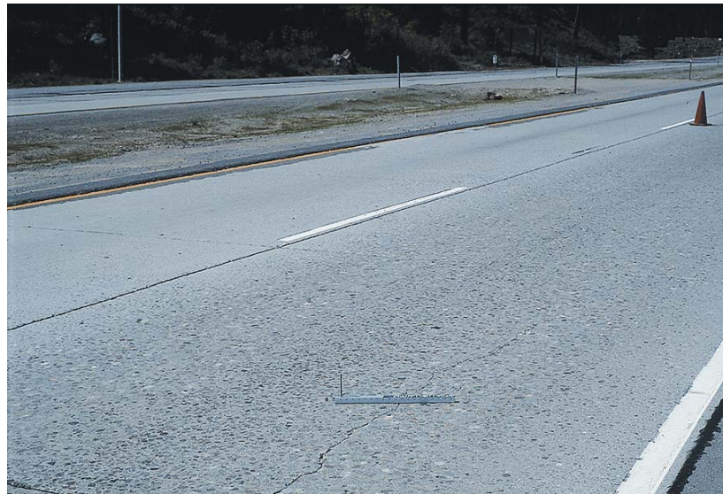
Figure 39 - Low Severity Longitudinal Cracking
