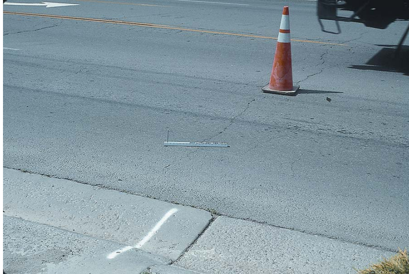
Figure 18 - Moderate Severity Transverse Cracking
