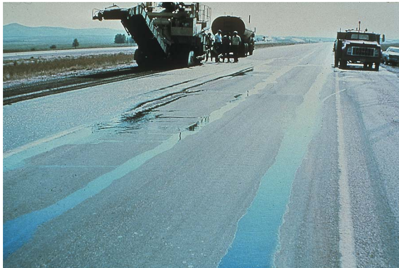
Figure 22 - Standing Water in Ruts
