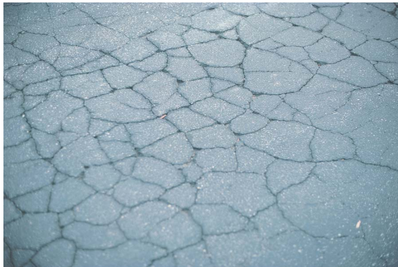
Figure 2 – Chicken Wire/Alligator Pattern Cracking
