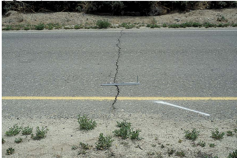
Figure 19 - High Severity Transverse Cracking
