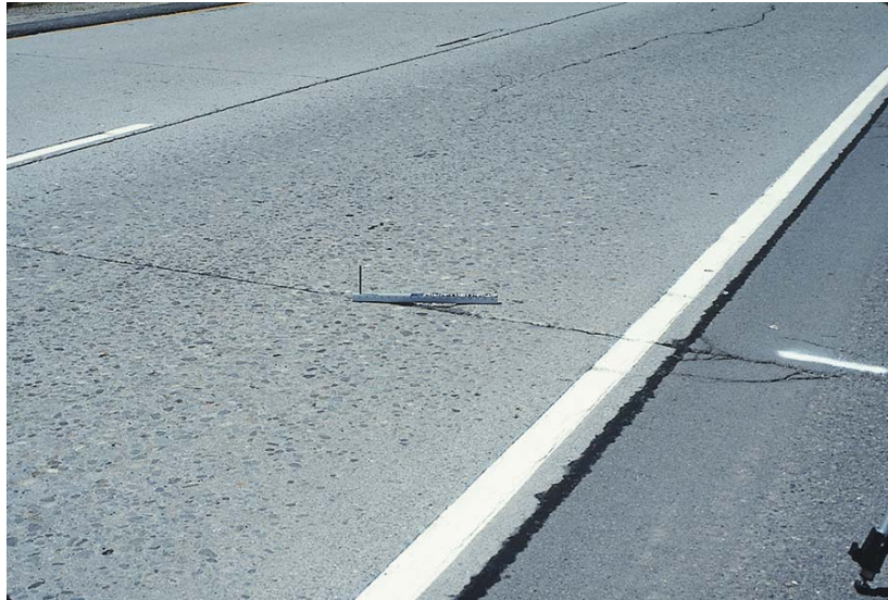
Figure 50 - Moderate Severity Spalling of Transverse Joint, Far View
