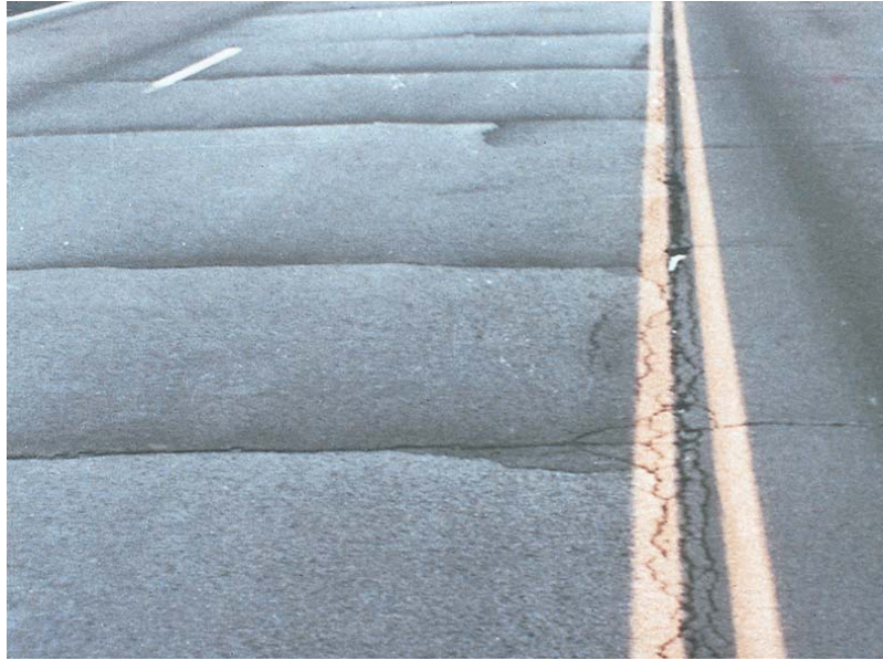
Figure 15 - High Severity Reflection Cracking at Joints
