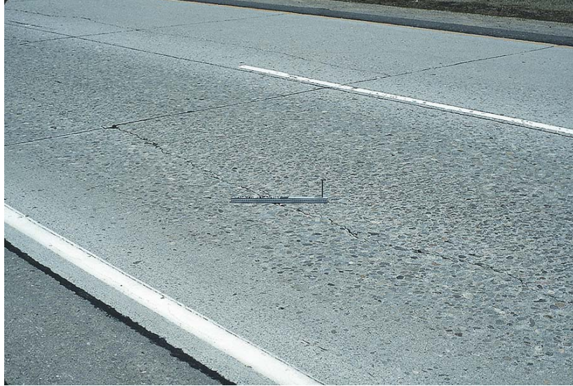
Figure 40 - Moderate Severity Longitudinal Cracking
