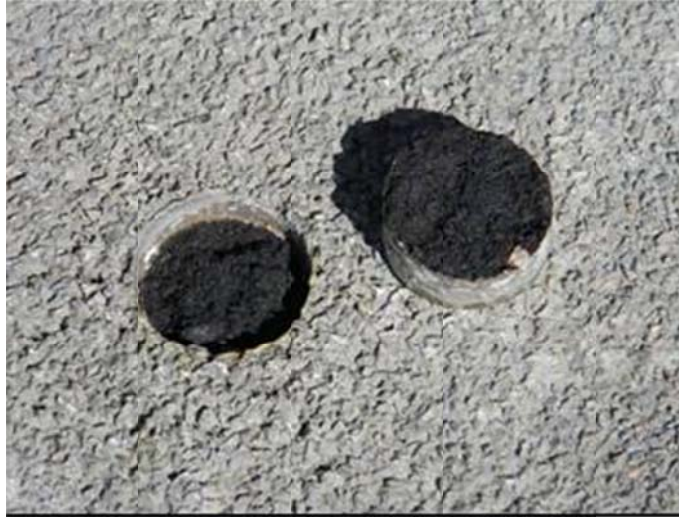
Figure 5.2.3.5: Failure of the Asphalt Under SafeLane Overlay
