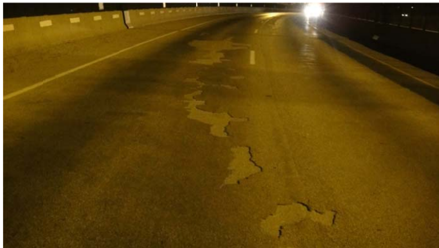
Figure 7.1.1.4 Delaminated Flexogrid Overlay
