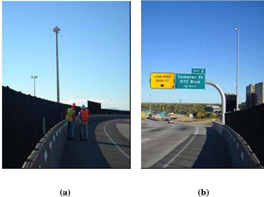
Figure 5.1.3.4: Sensor Masts on I-25 / I-225 (a) Infrared, and (b) Camera
