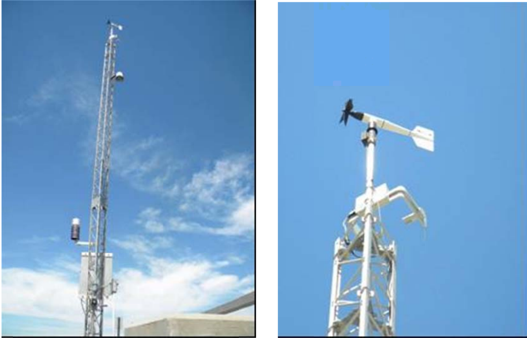
Figure 5.1.1.4: Weather Station at I-76 / WCR-53
