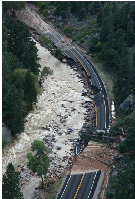
Flooding caused severe damage to state and local roads. Although some of the most extensive damage occurred to roadways through mountain canyons (left), as flood waters moved east, roads and bridges in the plains were impacted as well. SH 66 is shown below.
