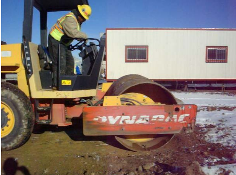
Figure 10. Single drum roller (73-kN) used to compact ESR layers in the field
