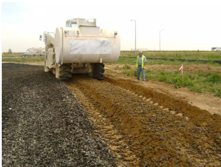
Figure 9. Rotary tiller typically used in lime/fly ash stabilization employed during field construction of an tire chip-ESR stabilized subgrade layer
