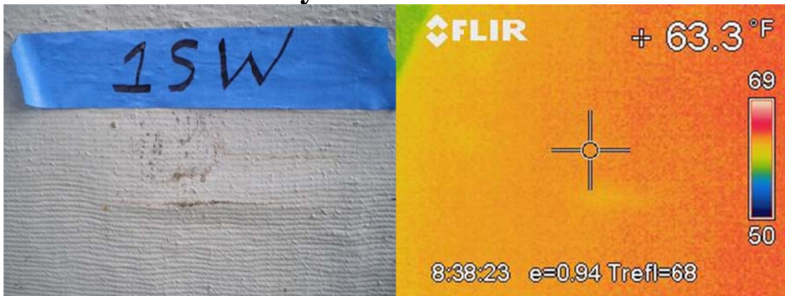
Figure A24. Photograph and thermal image of a defect found in Bay 1SW
