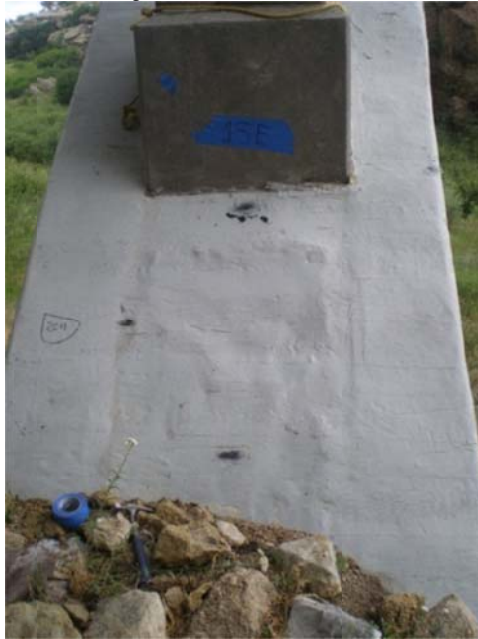
Figure A23. Bay 1SE, 1 void
