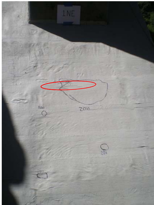
Figure A4. Bay 1NE, 4 of the 5 voids; crack exists, enclosed in red oval, in the top of the largest void
