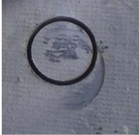
Figure 3.4. Damage caused by core bit without the use of the jig
