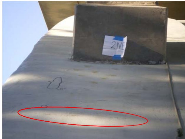
Figure 2.16. Crack identified in 2007
