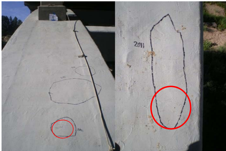
Figure 2.14. Outlined in permanent marker are identified areas of debonding between the FRP and the substrate developed in the structure between inspections in 2007 and 2011. Faintly denoted in the bottom of the photographs (enclosed in red circles) are previously found voids identified with “DELAM 07” and lines distinguishing the boundaries of the voids.
