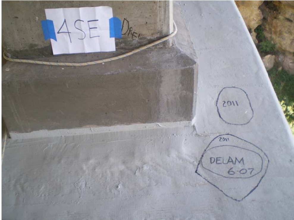
Figure A17. Void from 2007 has grown and a new void developed
