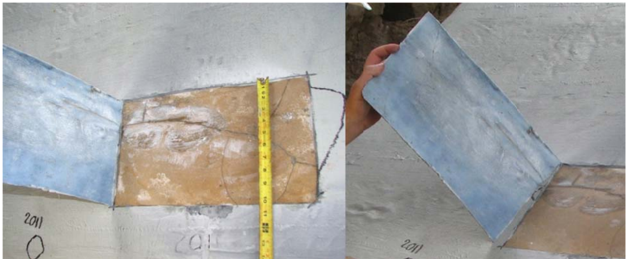
Figure 3.22. Cracks in the substrate were transmitted through the CFRP and notice the smooth texture and blue and white color of the underside of the CFRP
