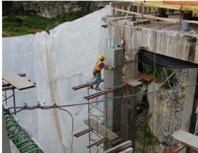
Figure 2.7. Placing the new spandrel columns adjacent to the existing columns (Mohseni, CDOT)
