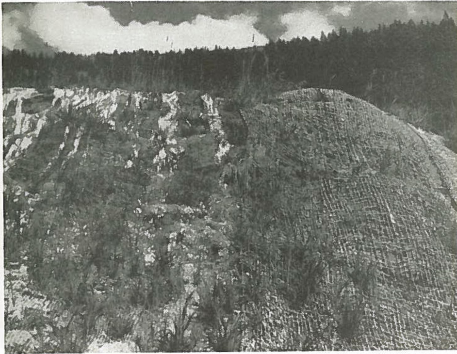
Photo No. 7 Taken 9/12/78 Vail Pass Hold-Gro, Sta. 654+50 Installation Date: 8/25/77 Hold-Gro on left, standard jute on right. Rocky knoll at top of medium fill slope.
