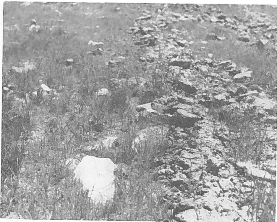
Photo No. 4 Taken 6/27/78 Same site as Photo No. 1. Rock and mud slide deposit is visible on right side. Hold- Gro paper has disappeared completely.
