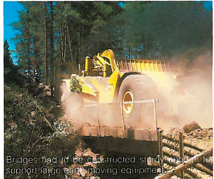
Haul bridges were constructed of timbers to minimize stream side disturbance and protect existing water quality during bridge dismantling after construction is completed.
