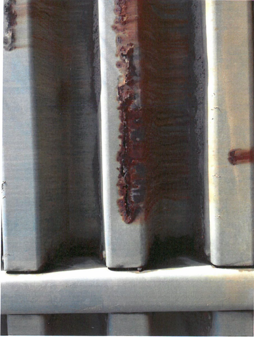
Deterioration of the existing crib wall
