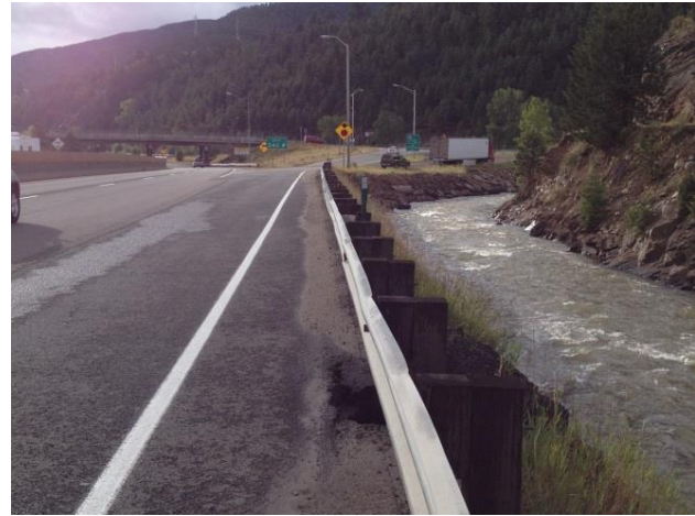
Example area where direct runoff from eastbound I-70 may flow directly into Clear Creek. (SH 103 off-ramp)
