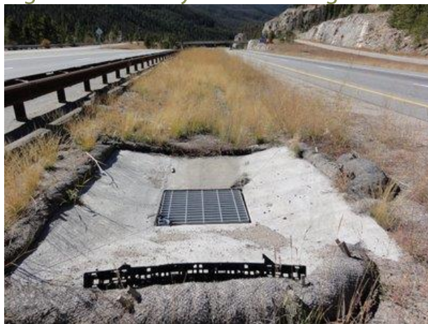
Inlet capturing runoff from both traffic directions.
