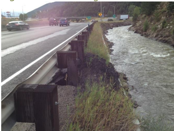
View along eastbound I-70 showing backfill loss at at SH 103 retaining wall.
