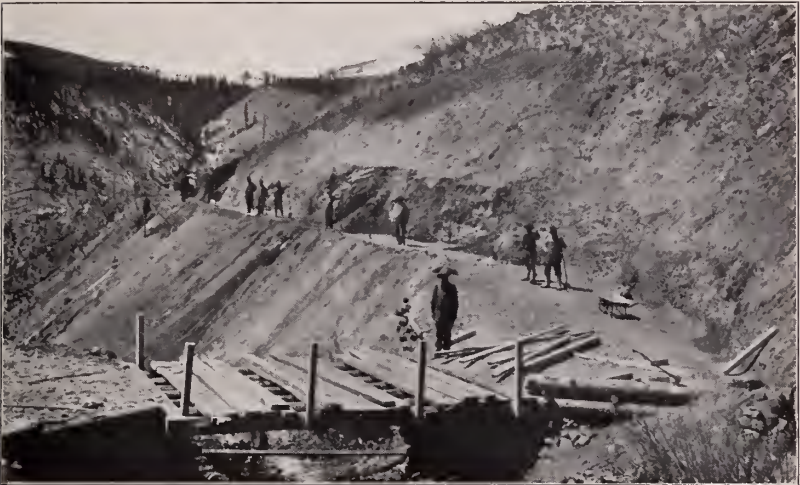
Road Building, Near Crested Butte, Gunnison County, Colorado. Work Prosecuted Under Supervision of Committee
