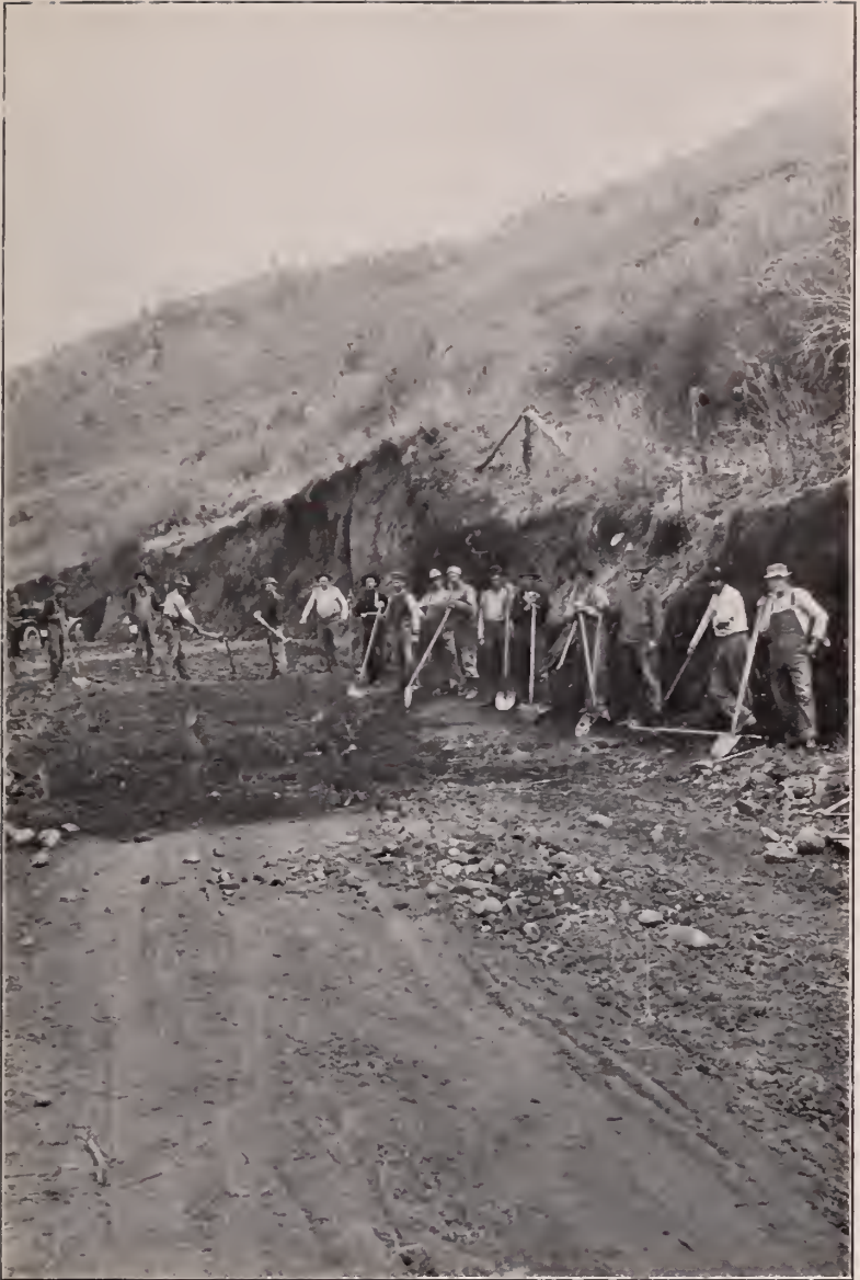
Rebuilding Road in St. Vrain Canon, Boulder County, Colorado. Work Prosecuted Under Supervision of Committee
