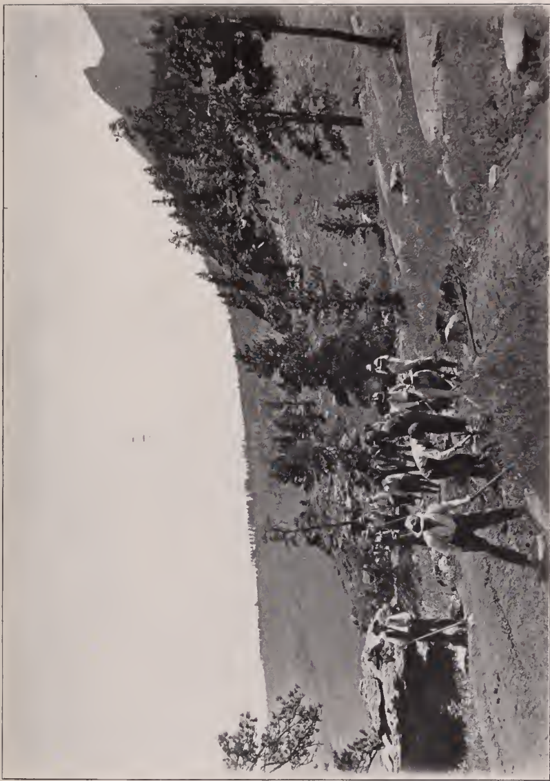
Rebuilding the Flagstaff Road, Near Boulder, Colorado. Work Prosecuted Under Supervision of Committee
