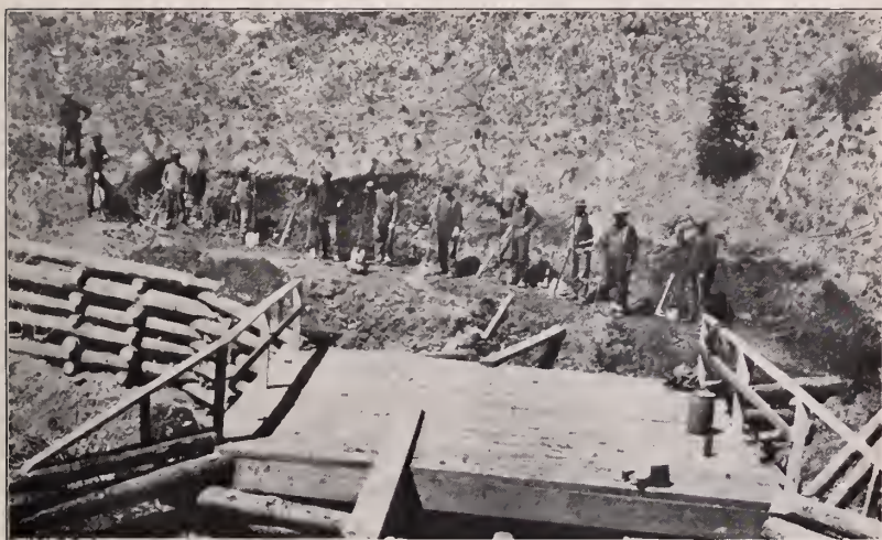
Road Building, Near Crested Butte, Gunnison County, Colorado. Work Prosecuted Under Supervision of Committee
