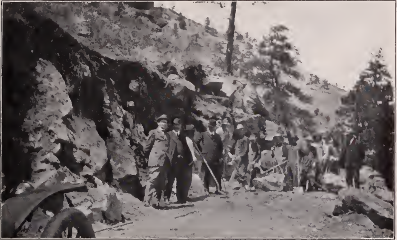
Rebuilding the Flagstaff Road, Near Boulder, Colorado. Work Prosecuted Under Supervision of Committee
