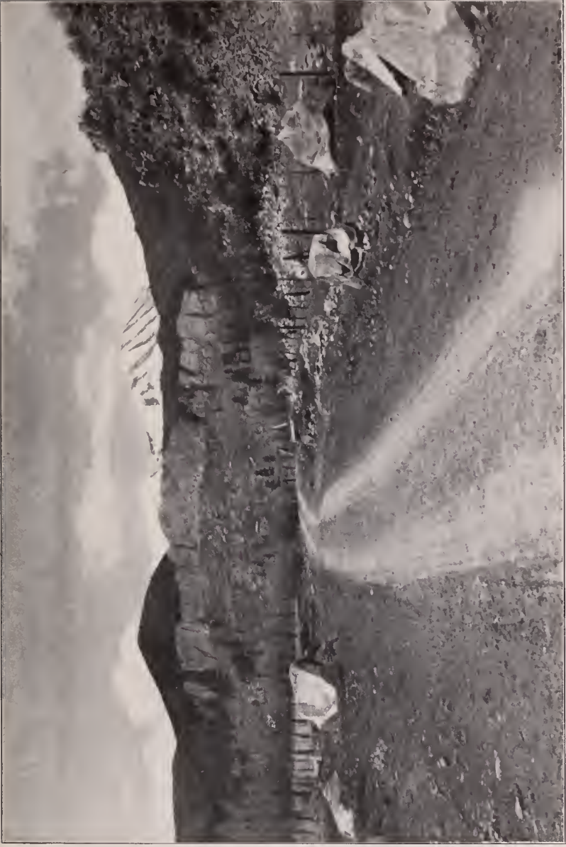
The Same Section of the Stonewall Road Completed. Observe the Snowy Range in the Background
