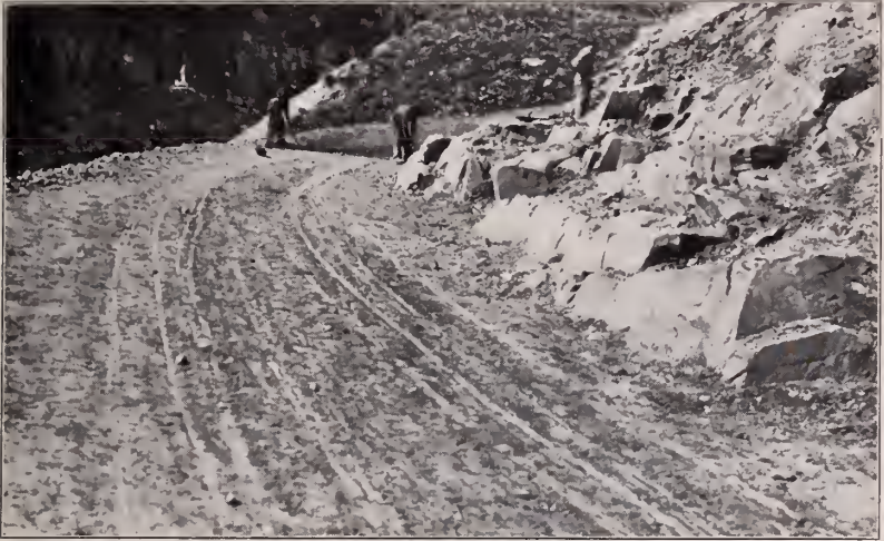
Finishing a Section of Road in Crested Butte Region, Gunnison County, Colorado. Work Prosecuted Under the Supervision of the Committee
