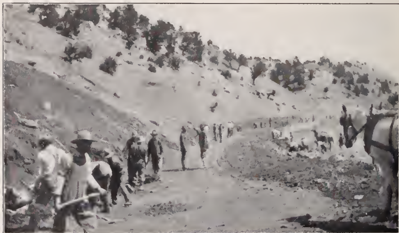
Finishing a Section on Stonewall Road. Work Prosecuted Under Supervision of Committee
