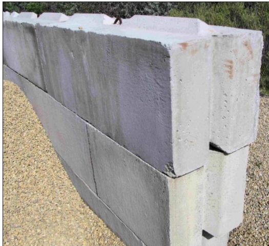
Figure 2-2. Stacked blocks form retaining wall. The rebar hook in the top middle enables manipulating blocks with a back hoe or similar farm tool.
