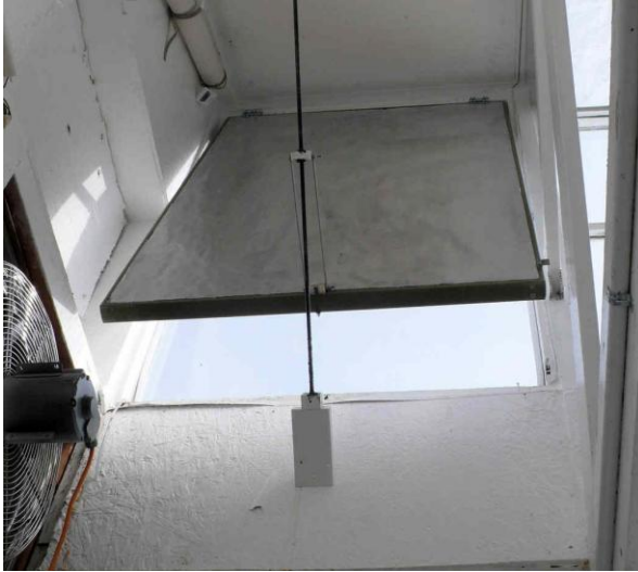
Figure 3-11. #1 upper shutter on the far east end of the greenhouse about 20 percent open. Note adjacent exhaust fan and air intake near the top of the shutter.
