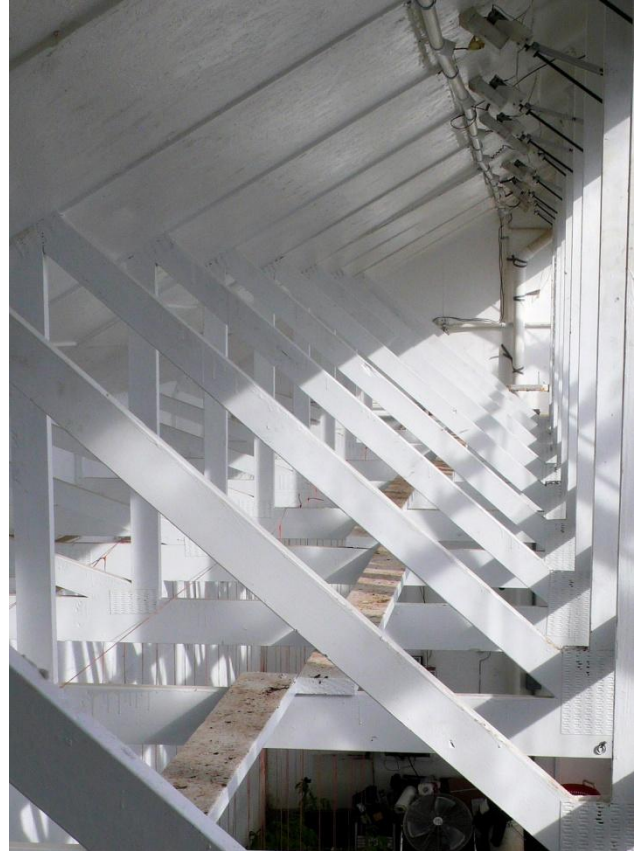
Figure 3-12. View from the trusses looking east, swinging shutters open, gear motors at top.
