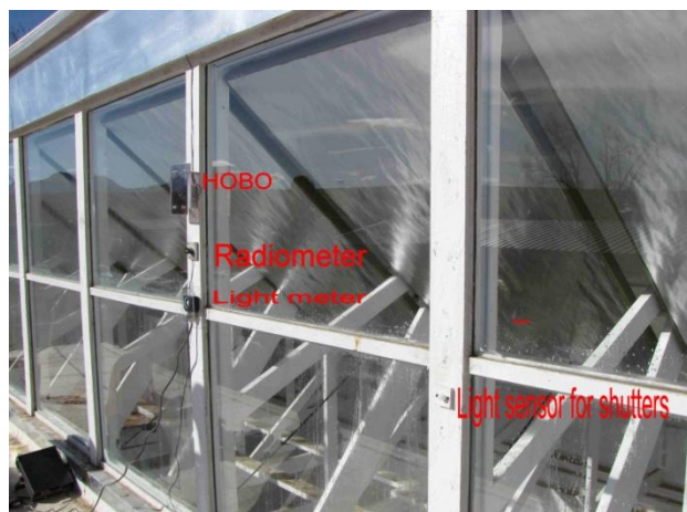
Figure 3-16. Center of roof with HOBO and other sensors.
